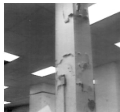
Deteriorating lead-based paint recorded in the OIG's first video report concerning a Postal facility.
