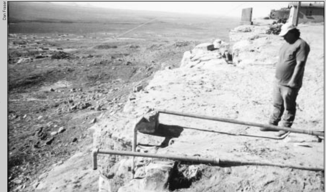
Chuck Villa, water system operator, looking down at the exposed transmission main ascending the face of the cliff.
