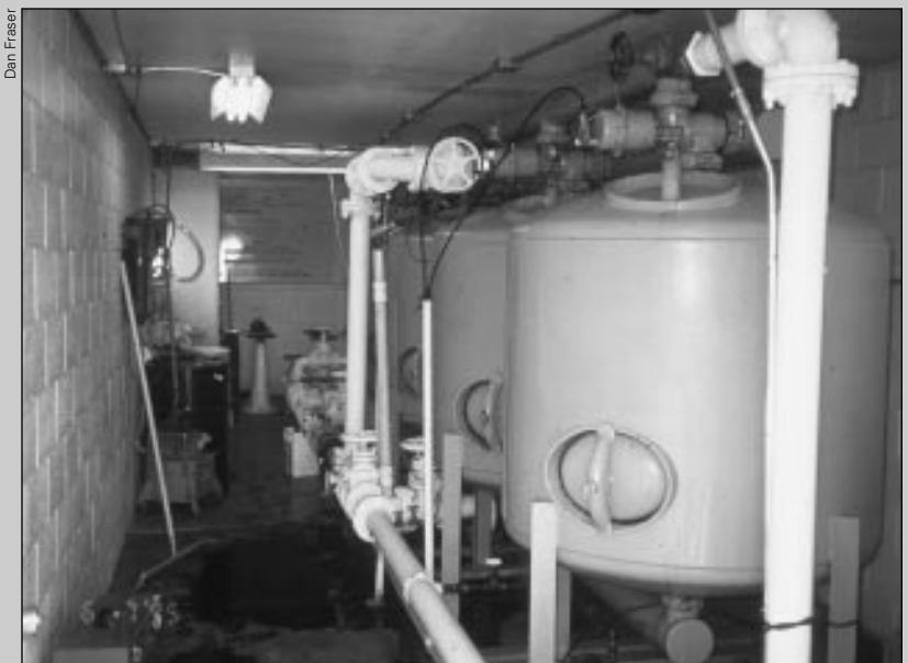
Pressure filters at Ethete
