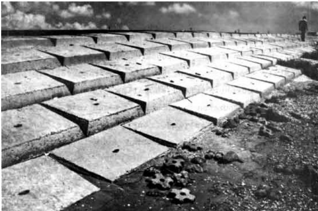
Figure 24. New revetment installed to protect the shoreline and Highway 82 in Cameron Parish, LA.
