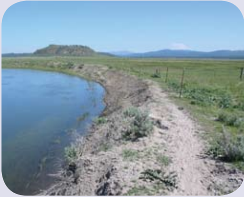
The river levees on the C7 ranch will be removed, reconnecting the river to its nature floodplain.
