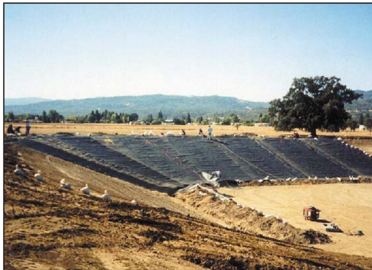
Installation of a liner at the Round Valley Reservation Wastewater Treatment Lagoon
