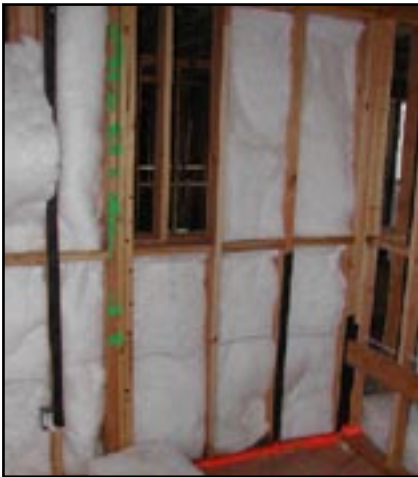
Materials: Batt insulation
