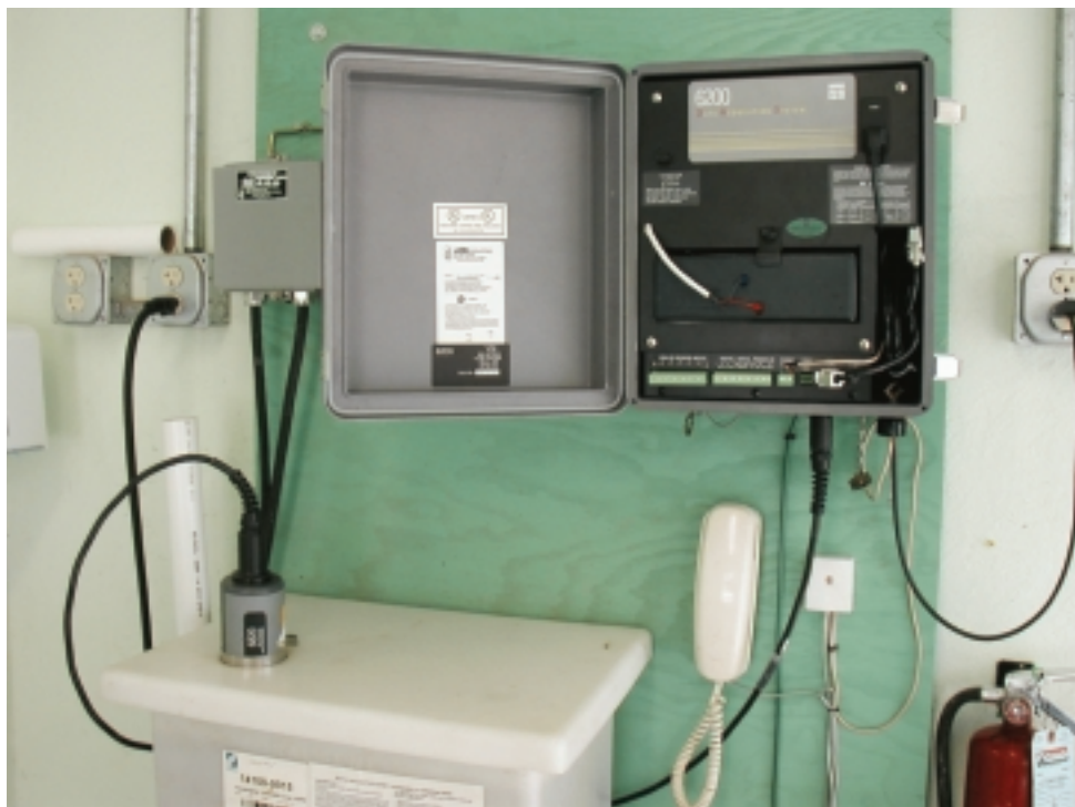
Figure 14. Data acquisition system at Downtown Dayton monitoring station
