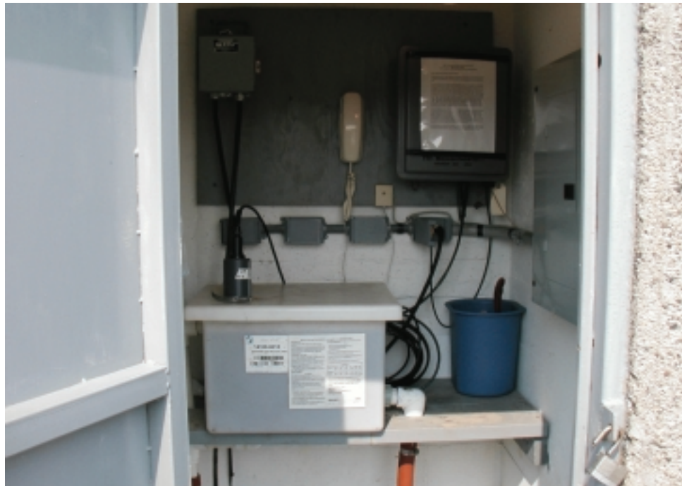
Figure 6. Flow-through Tank at the Wolf Creek Monitoring Station
