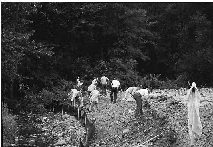
Save Our Streams volunteers working together to lay a facine in a trench. Credit: Jay West
