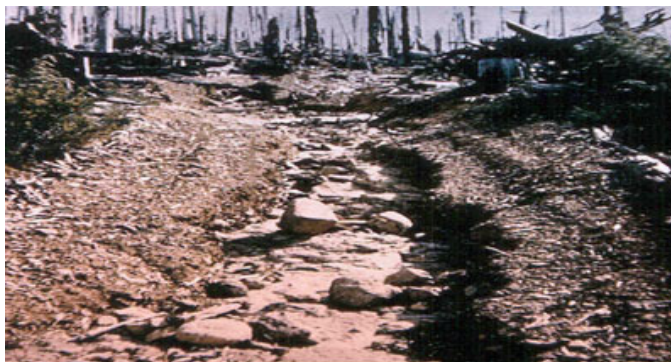
This improperly sited and maintained logging road has eroded badly and essentially functions as a new intermittent stream. Drainage ditches of properly maintained roads also can increase stream density and reduce groundwater recharge.
