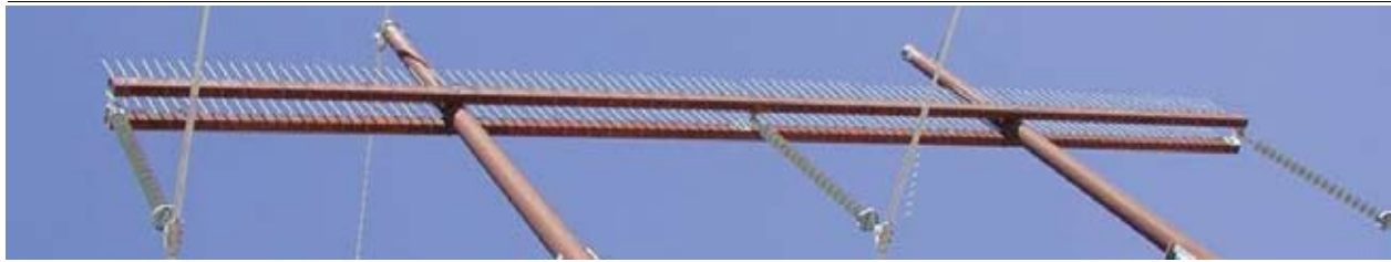
Figure 3. Perch-deterrent devices installed on surveyed, power-line structure.
