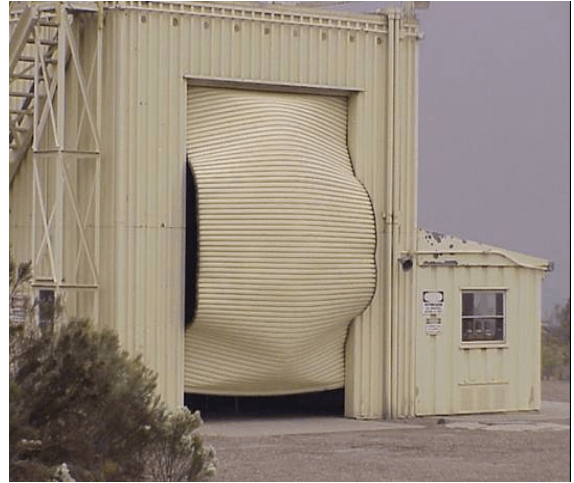
Picture 3. Severely damaged inflation shelter at Upper Air Facility. Courtesy of WFO San Diego.
