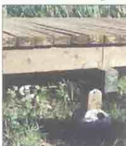
Photographs of the Pin Foundation Diamond Pier and boardwalk from the Nisqually National Wildlife Refuge.
