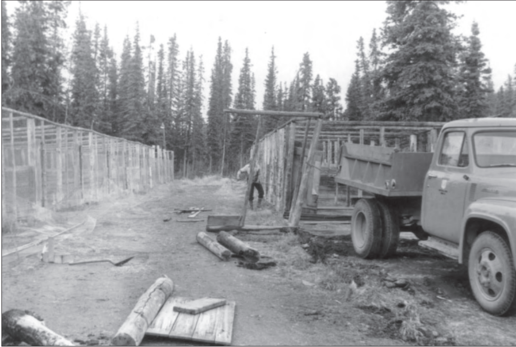
Figure 1.65. View west of the dog kennels during renovation, October 1955 (DENA 11-40, Denali National Park and Preserve Museum Collection).
