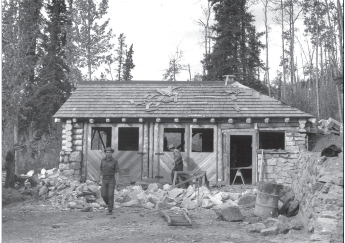
Figure 1.40. View west of CCC enrollees at work during construction of the superintendent's garage (Building 111), 1939. Note the retaining wall (111A) on the right (DENA 3-5, Denali National Park and Preserve Museum Collection).
