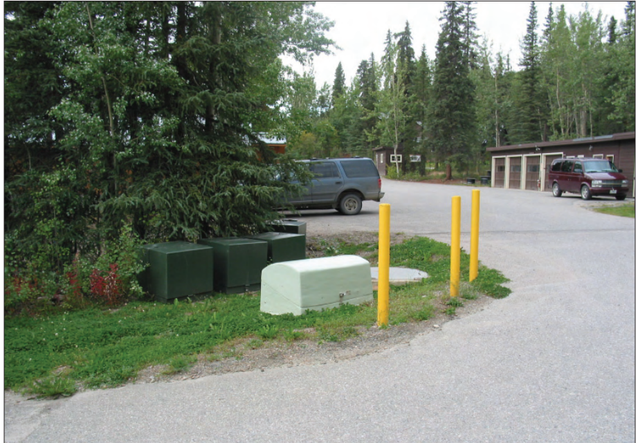
Figure 4.42. Small-Scale Features - Replace prominent safety bollards with appropriate rustic measures - Treatment Task 1.B - Replace non-historic steel bollards and otherwise visually prominent safety barriers with non-historic alternatives that are consistent with the historic character of the landscape. In this view of existing conditions, the visual prominence of both the barriers and the utility features detract from the rustic character of the landscape (OCLP, 2006).
