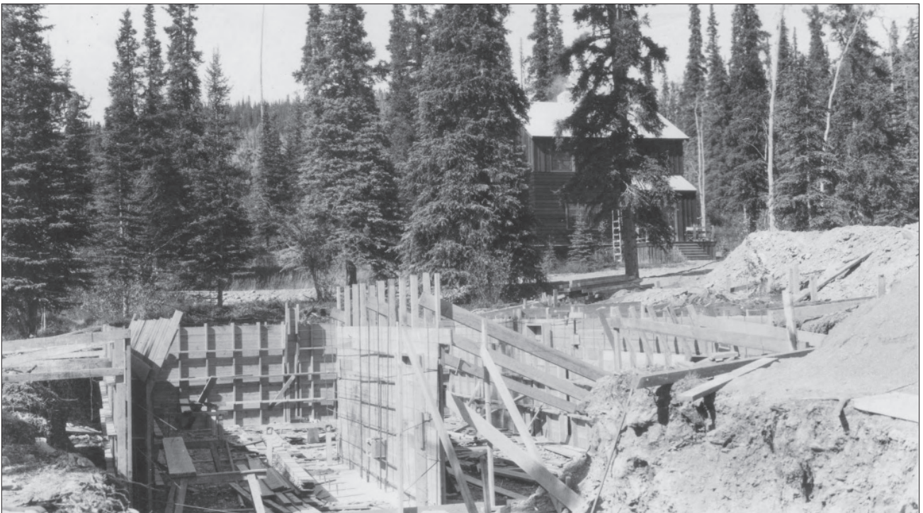
Figure 1.46. View northwest of concrete forms in place for construction of the new employee's residence basement (Building 23), August 1940. Depicted in the background is one of the two employee residences built in 1939 (Building 13) (National Archives and Records Administration, College Park, MD).
