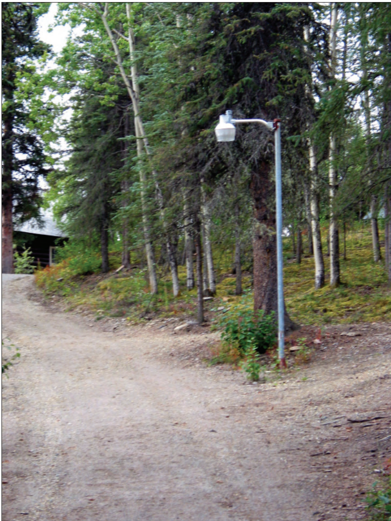
Figure 2.16. Light fixture in headquarters area, south of of Building 112 (August 2005, OCLP).
