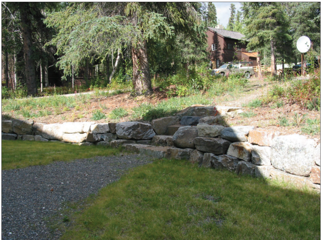
Figure 3.32. View west Bldg. 23 (original employee's residence) of a recently constructed stone retaining wall and steps (August 2005, OCLP).
