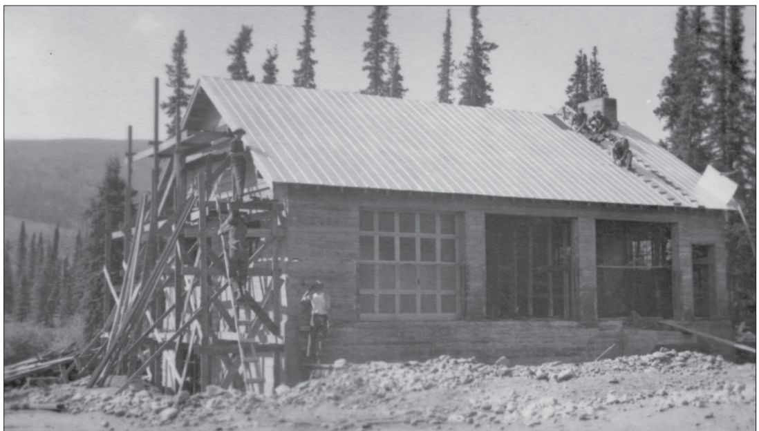
Figure 1.41. View southwest of the machine shop and garage (Building 102), June 28, 1939 (DENA 3-1, Denali National Park and Preserve Museum Collection).
