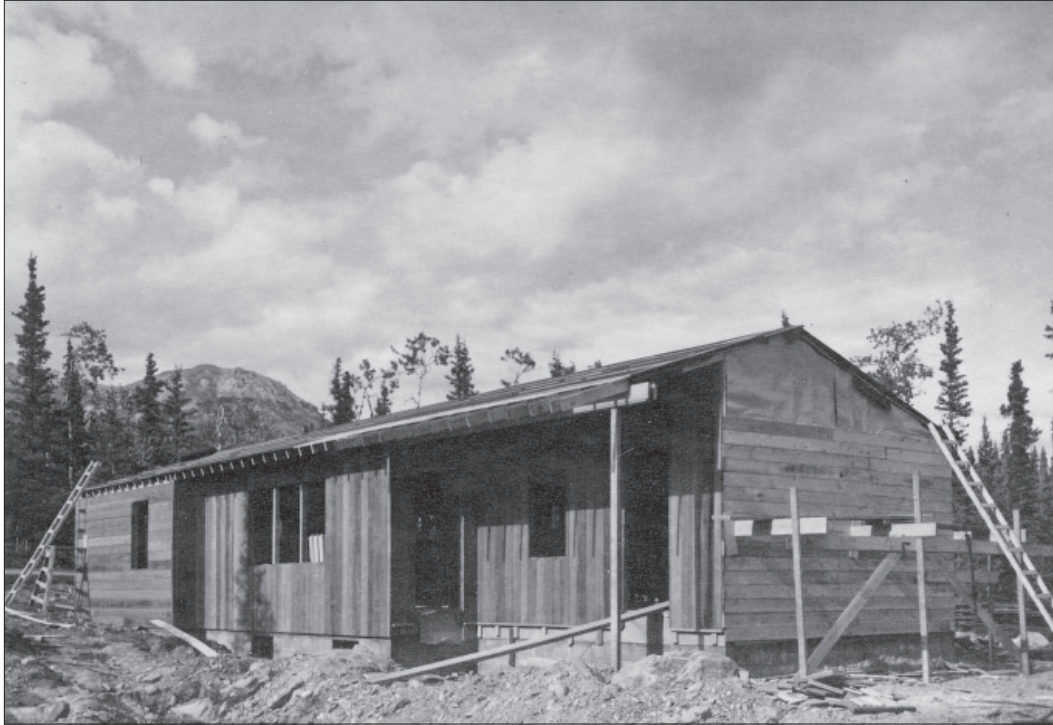
Figure 1.59. Employee's residence (Building 26), designed by regional architect Cecil Doty, under construction, July 21, 1950 (NPS, Alaska Regional Office, CLI program files).
