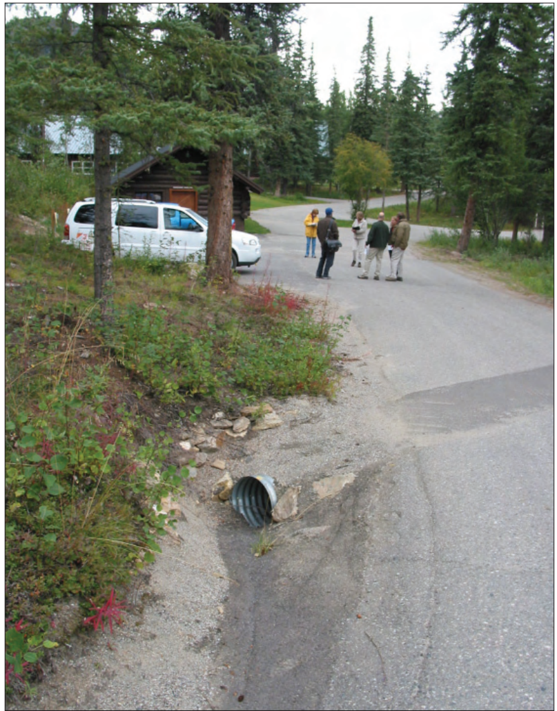
Figure 2.5. The roads, paths and structures create a series of terraces within the headquarters area which retain water and are drained by culverts and swales. Inflow of culvert south of Building 107, Plumbing Shop (August 2005, OCLP).
