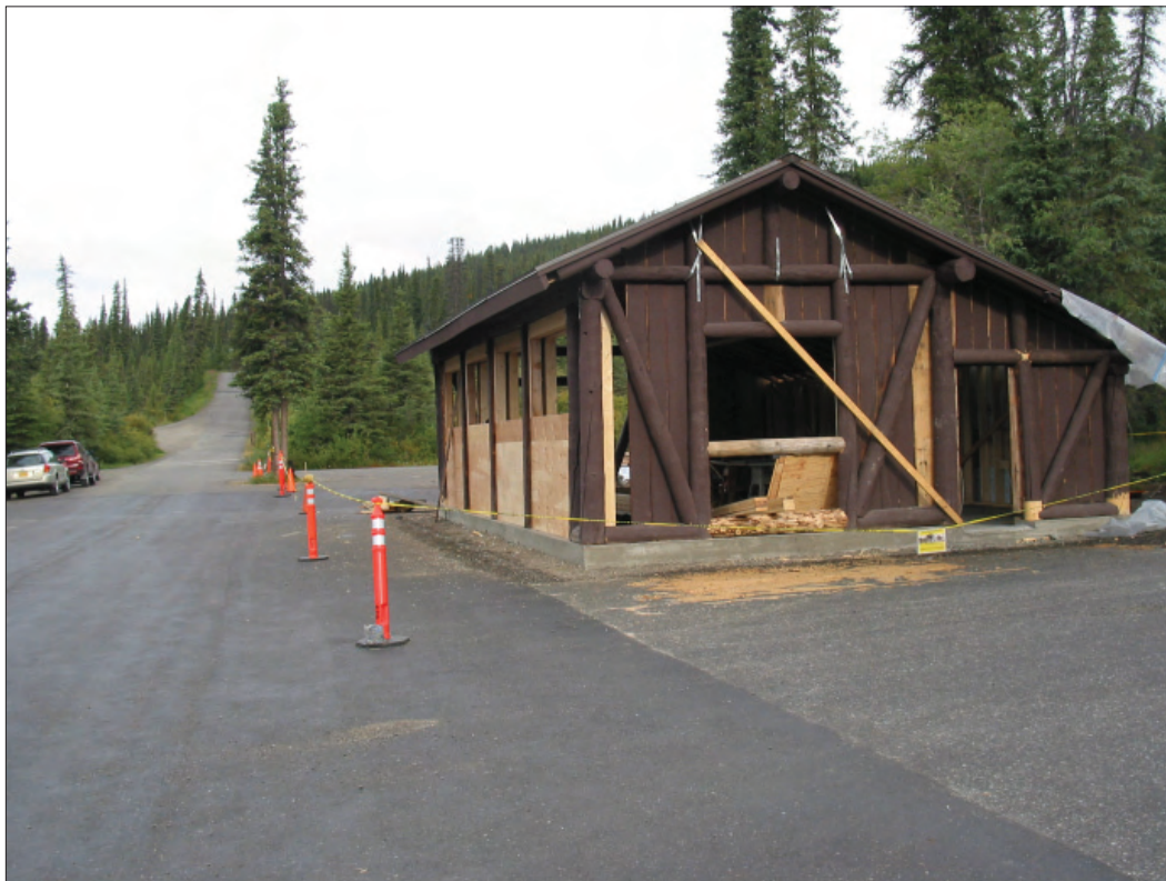
Figure 1.75. View west of original garage (Building 103) during rehabilitation (NPS, Olmsted Center for Landscape Preservation, 2006).
