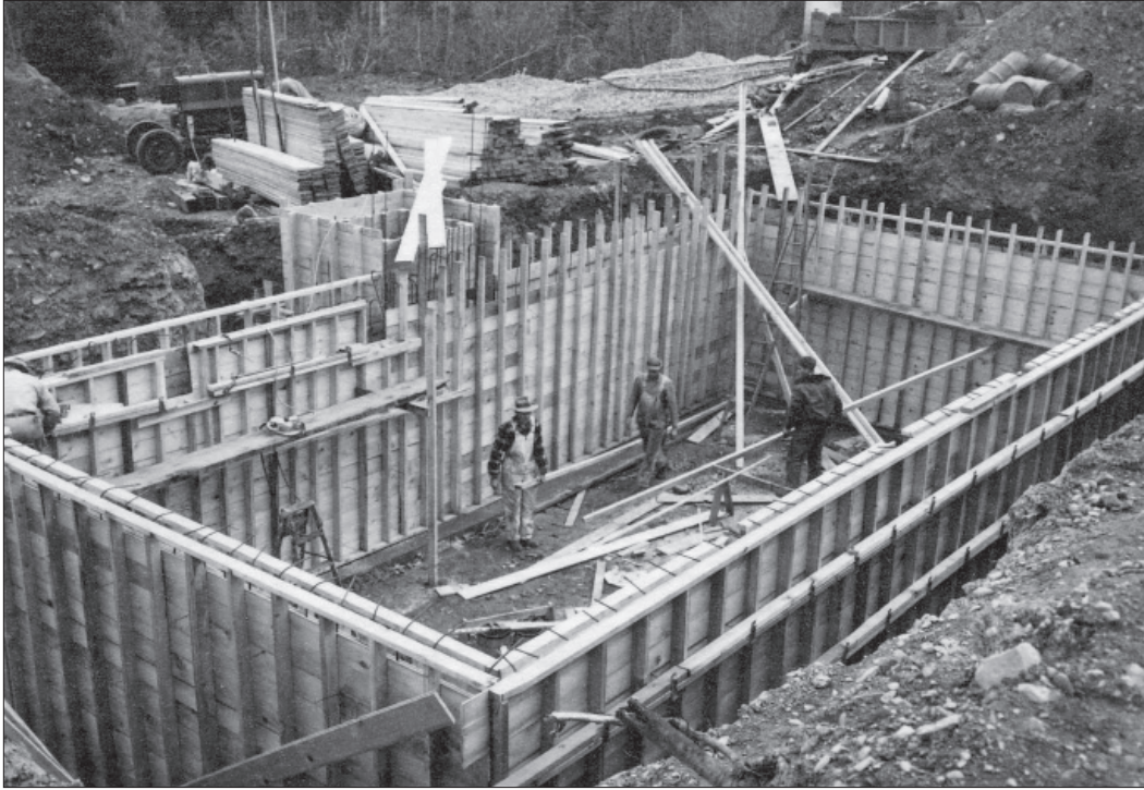
Figure 1.61. View during construction of the 50,000 gallon reservoir, September 26, 1950 (NPS, Alaska Regional Office, CLI program files).
