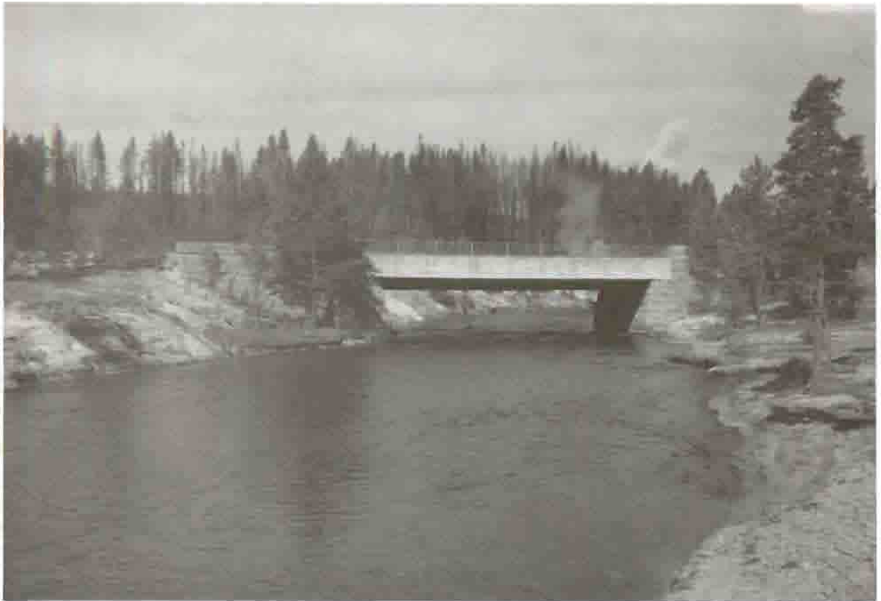
Firehole River Bridge, Near Morning Glory Pool, 1989 Courtesy Historic American Engineering Record, Jet Lowe, 1989
