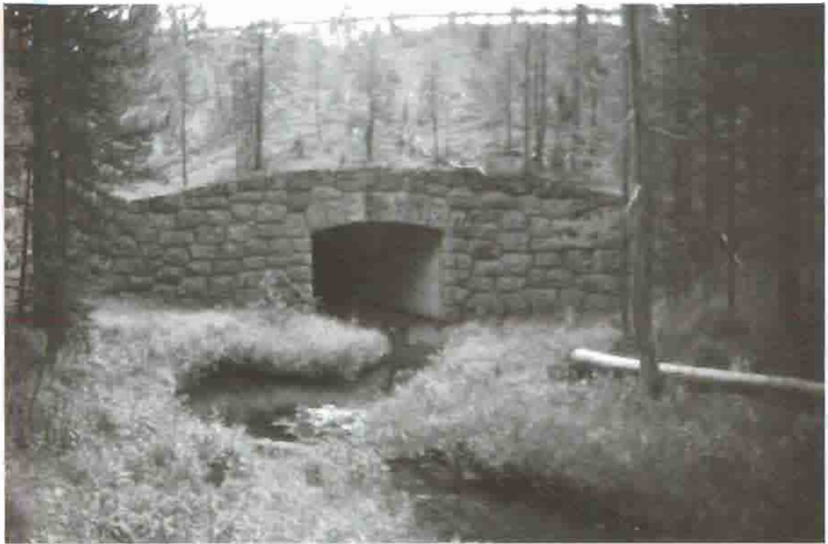
Culvert on Old Faithful to West Thumb Road, 1989 Courtesy Yellowstone National Park Archives
