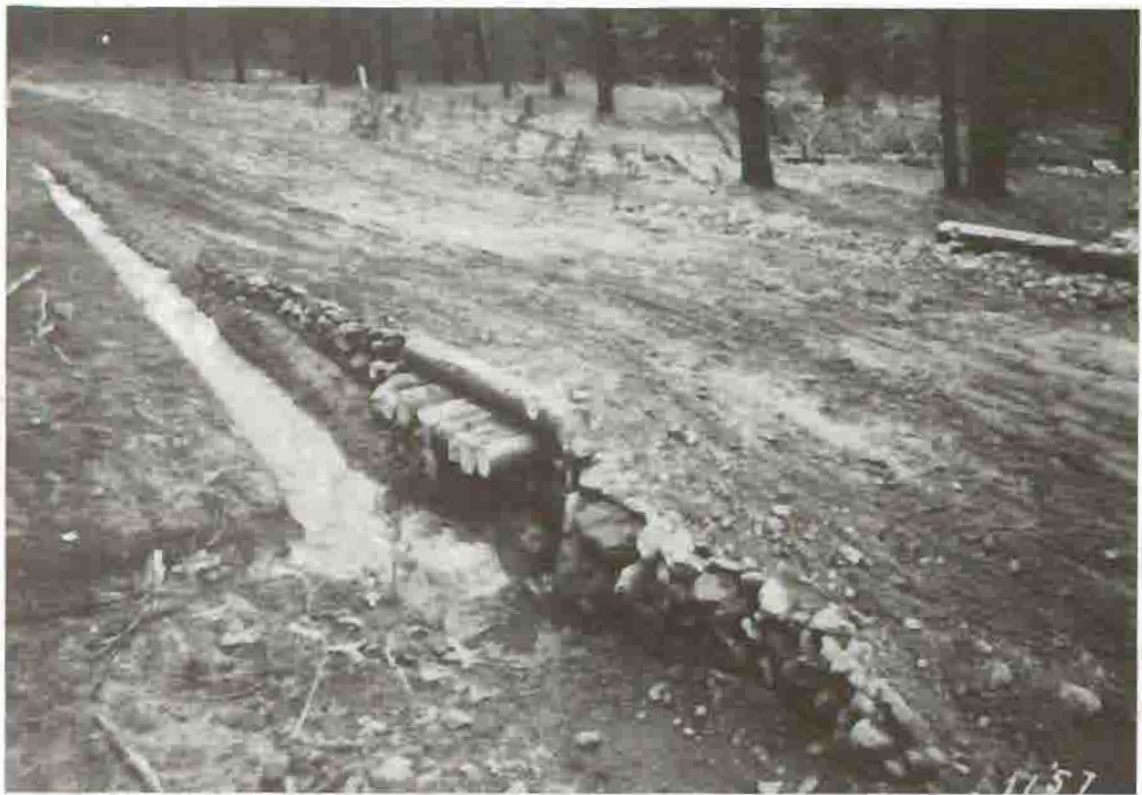
Culvert and Ditch Construction on Cooke City Road, United States Army Corps of Engineers Courtesy Yellowstone National Park Archives
