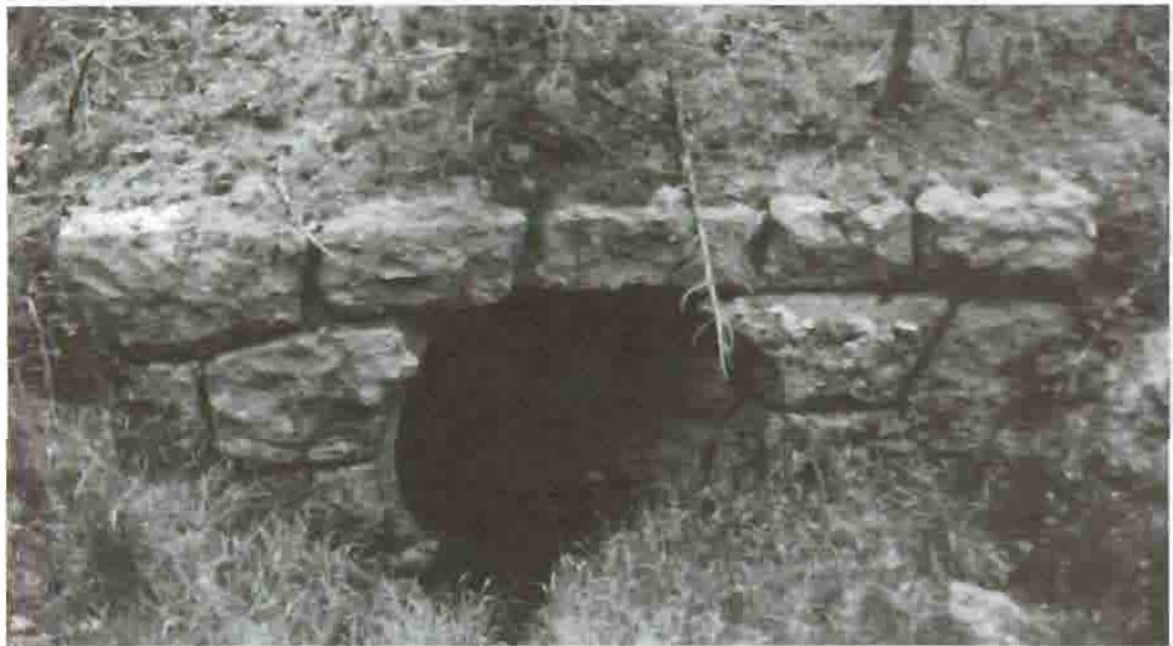
Culvert on Old Faithful to West Thumb Road, 1989 Courtesy Yellowstone National Park Archives
