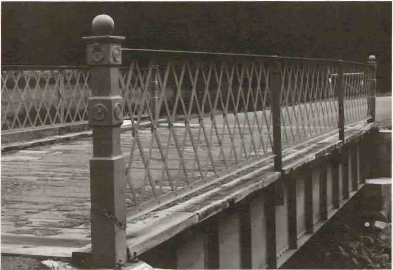
Detail of Obsidian Creek Bridge, 1989 Courtesy Historic American Engineering Record, Jet Lowe, 1989
