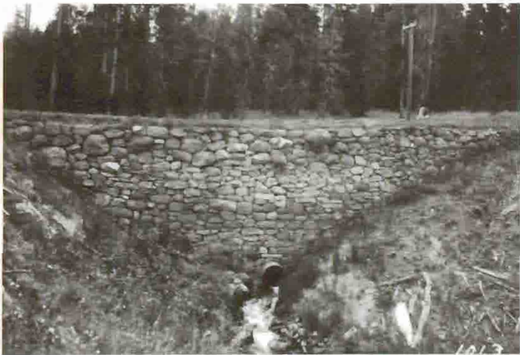
Retaining Wall Near 2 Milepost, Lake to Canyon Road, 1912 Courtesy Yellowstone National Park Archives
