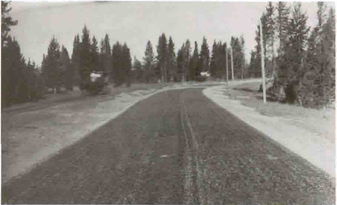
Completed Paved Road near West Entrance, United States Army Corps of Engineers Courtesy Yellowstone National Park Archives
