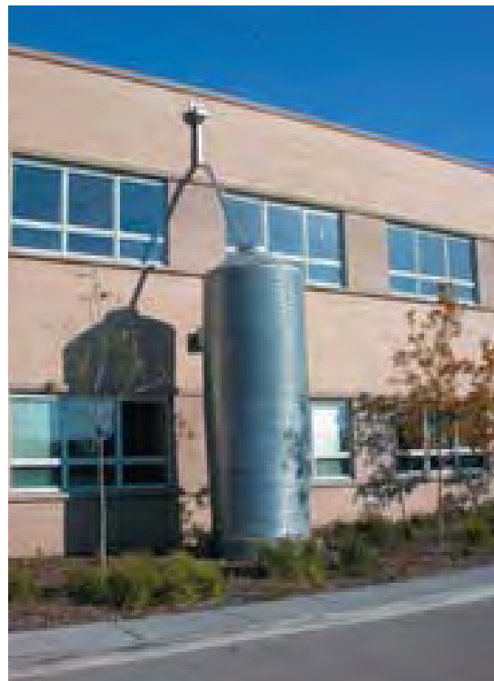
a cistern system collects rainwater from Chicago Center for Green Technology (Chicago, IL) (Photo: Conservation Design Forum)
