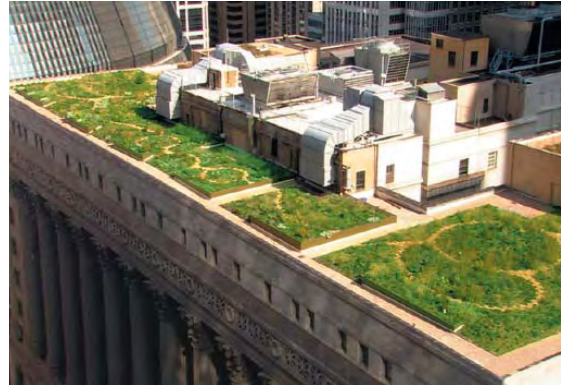
green roof (Chicago City Hall, IL) (Conservation Design Forum)
