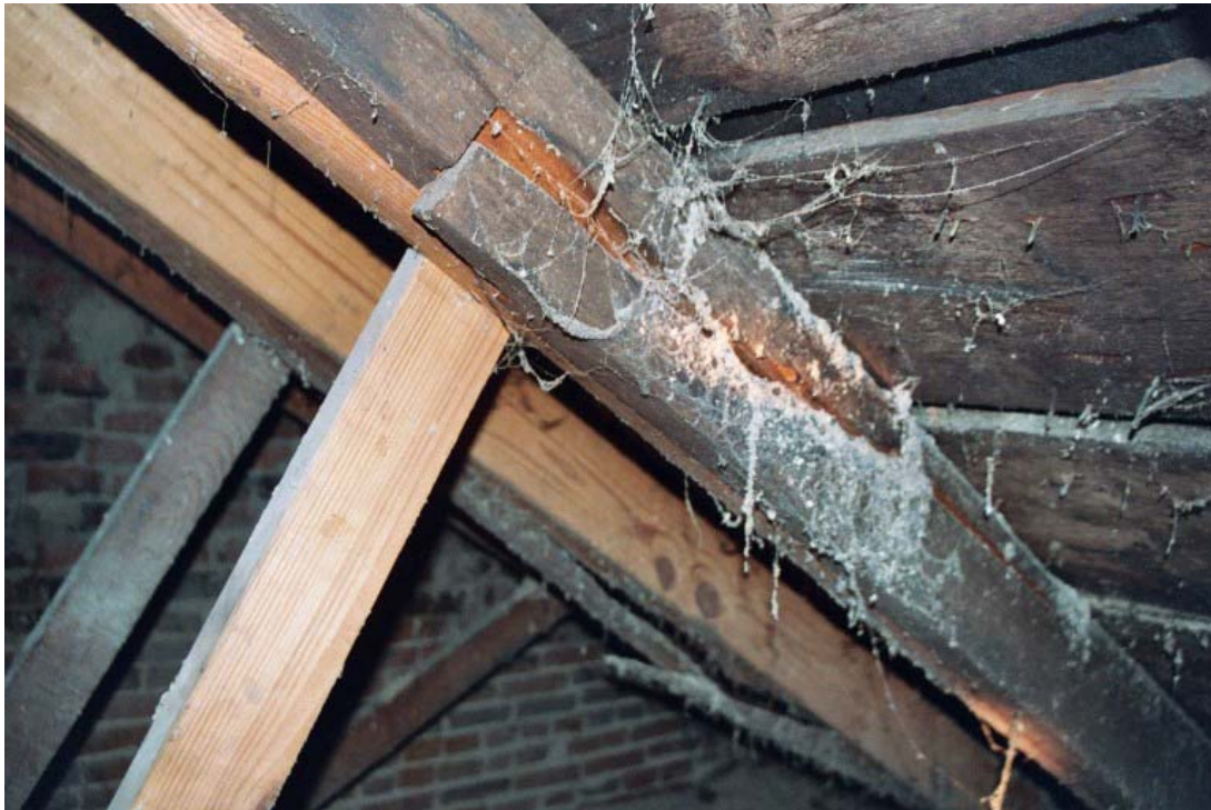
Figure 6 Fractured rafters near southwest chimney
