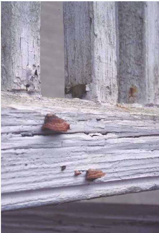
Figure C – 52 Fungus growing on the west porch balustrade
