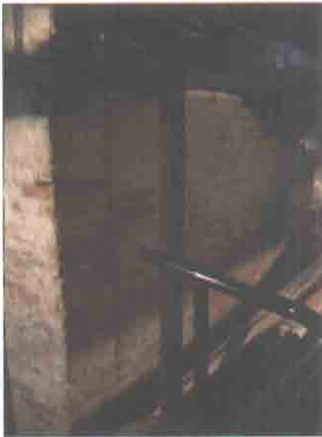
Figure 2.23. Room 001, view of unstable west wall of room 001a (central brick furnace chamber).
