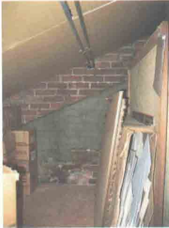
Figure 2.82. Room 307, looking west toward original brick gable end wall, showing roof line of 1864- 1865 addition and paint evidence.
