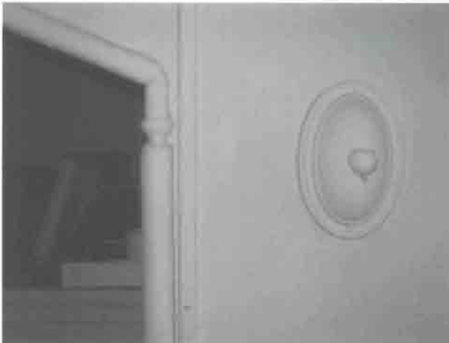
Figure 2.81. Room 306, wood corner guard on edge of recess, and remnant of light fixture.
