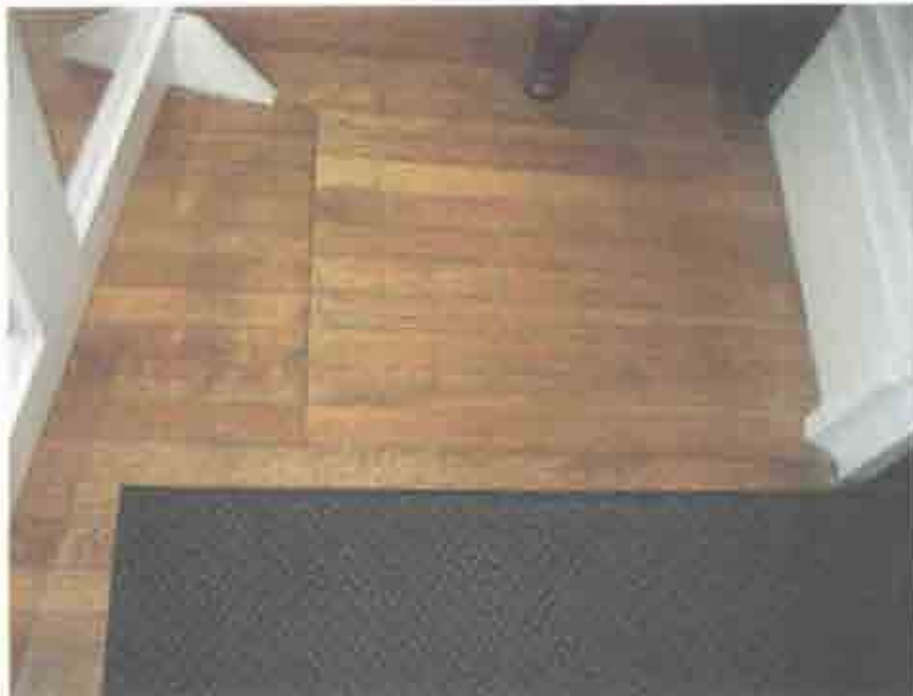
Figure 2.43. Room 108 (Dining Room), former location of missing floor register.
