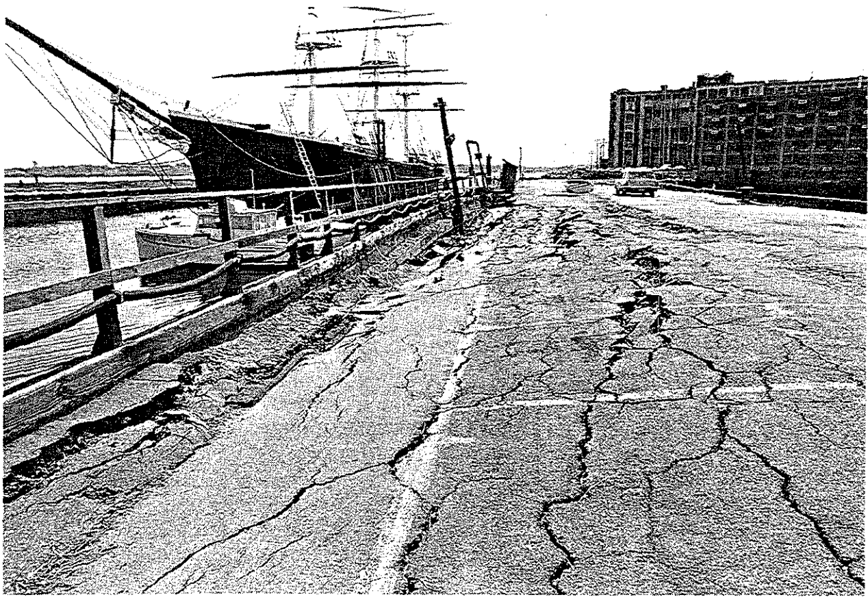
Figure 11. Central Wharf in 1972. Although visiting ships still occasionally tied up at the wharf, it was in need of extensive repairs due partly to neglect and partly to damage from construction of the Naval Reserve Facility. (Courtesy National Park Service, Harpers Ferry Center.)
