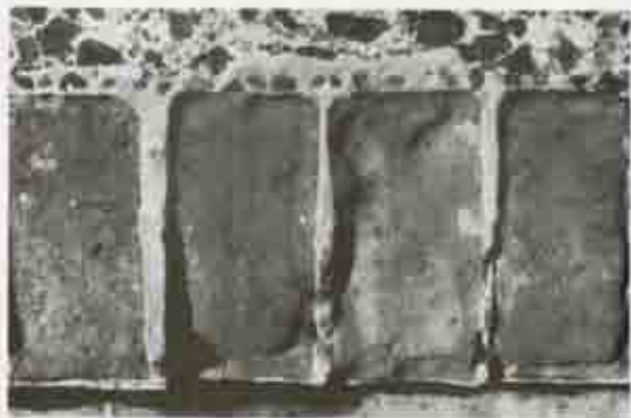
Figure 4. Northwest edge of ramp connecting the Plaza de Armas and Santa Barbara Battery. Brick galling is located between brick and concrete. Photo by J. Jacob, 1989.
