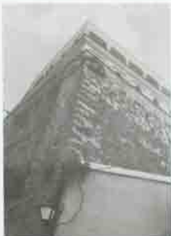
Figure 47. Saliest of Ia Concepción with missing sentry box, south wall. (Photo by R. Crissan, 1990.)
