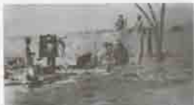
Figure 30. Nearly completed reconstruction of substructure at San Agustín Station. [West Wall], 1939. (SAJN HNS Archives.)
