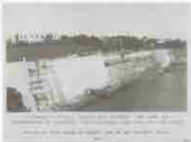
Figure 33. Curtain wall between Santa Elena and San Agustín Bastions, placing of stone facing on reconstructed wall, 1839. (SAJU NMS Archives.)
