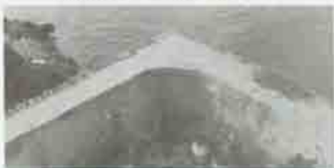
Figure 48. Southwest corner of Ia Concepción Bastion showing location of missing sentry box. (Photo by R. Crissan, 1990.)
