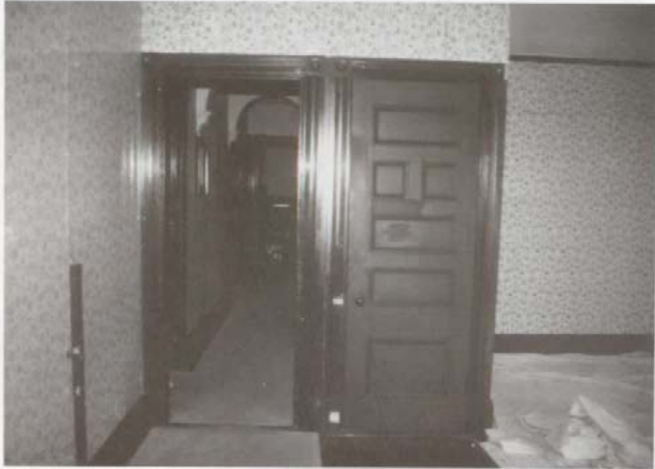
Typical Condition of Stained Woodwork
