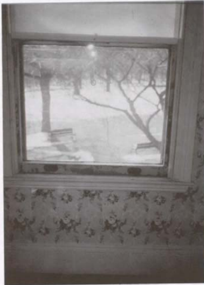
Typical Window Sash Condition Before Restoration
