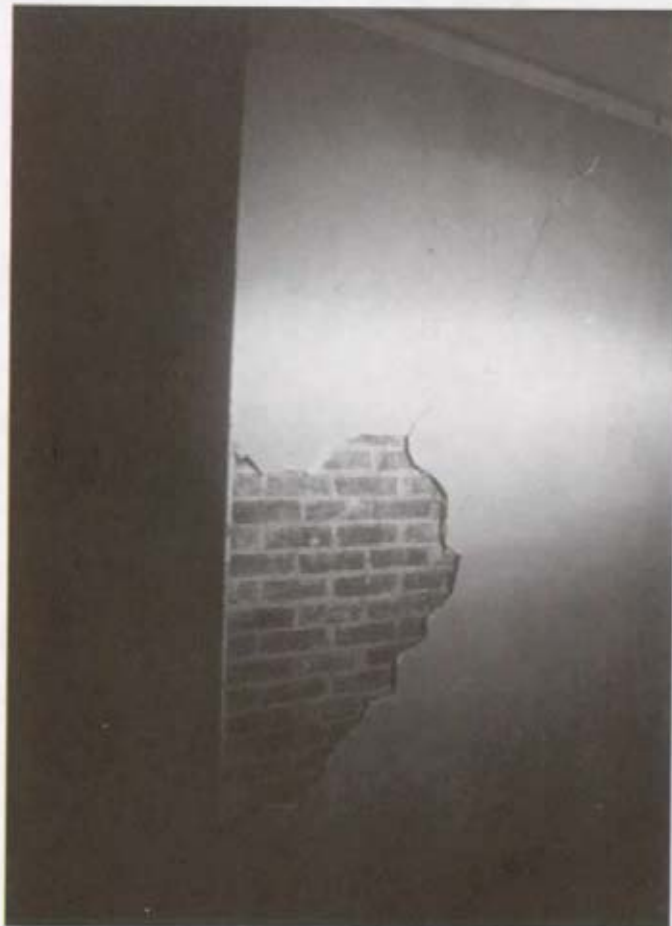
Alice's Room: Plaster Damage
