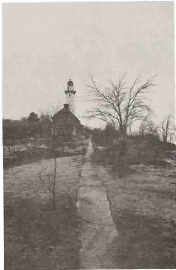
Illustration 24 Section of Concrete Walk Leading from Fog Signal House to Dwellings and Tower 1977
