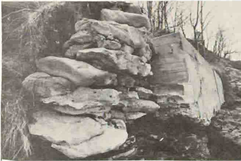
Illustration 31 Crumbling Section of Retaining Wall, Exposing Rock 1977
