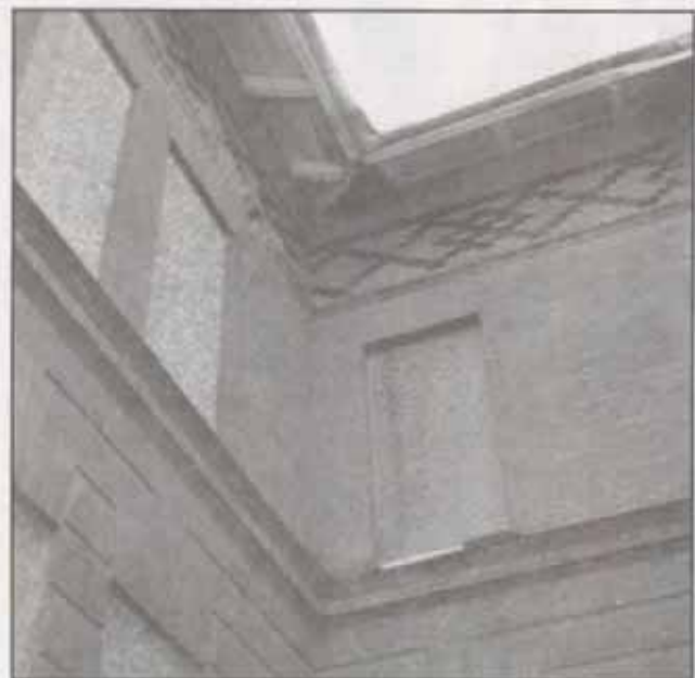
Figure 101. Detail, Vine Street School, showing wide eaves with beltcourse, and rusticated walls. Sebold.
