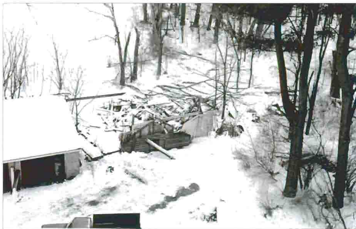
Figure 65: Birney garage, collapsed, 1977. Campbell's garage has been converted into a maintenance garage for the National Park Service. (MVB NHS).
