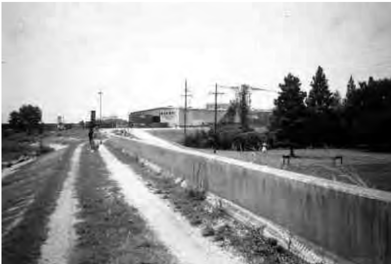
Figure 43. View along the levee crest, showing service lane and concrete wall that borders the landward edge of the crest.
