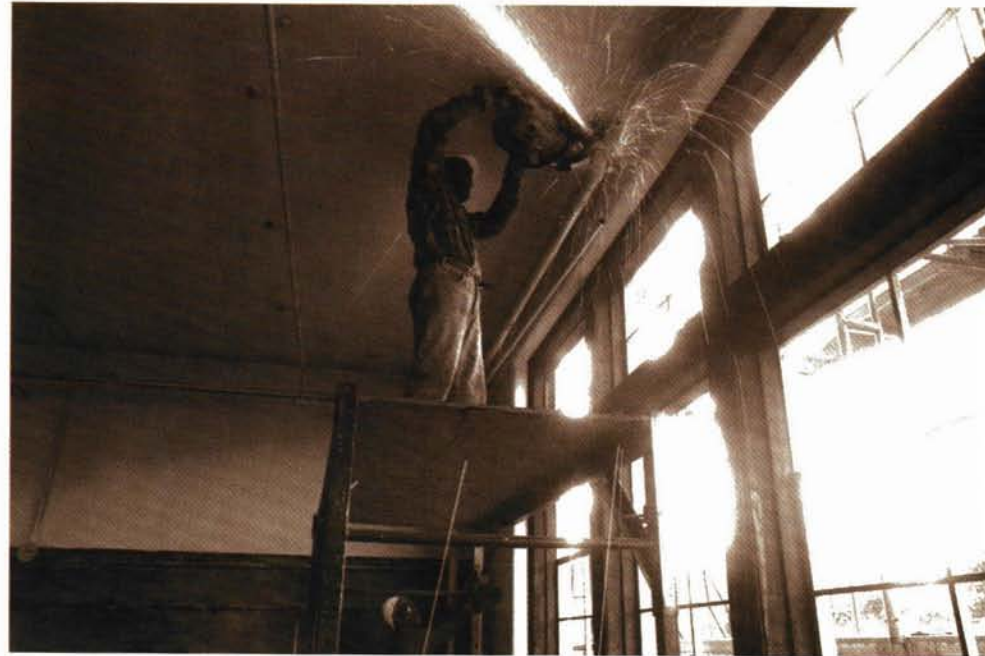
The Brandeis School in Louisville, Kentucky, was rehabilitated and transformed into housing through the use of the NPS Preservation Tax Incentives and the Low Income Housing Tax Credits. (New Directions Housing Corporation)
