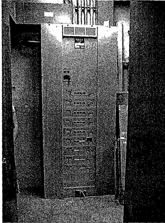
e: Main Electrical Distribution Panel
