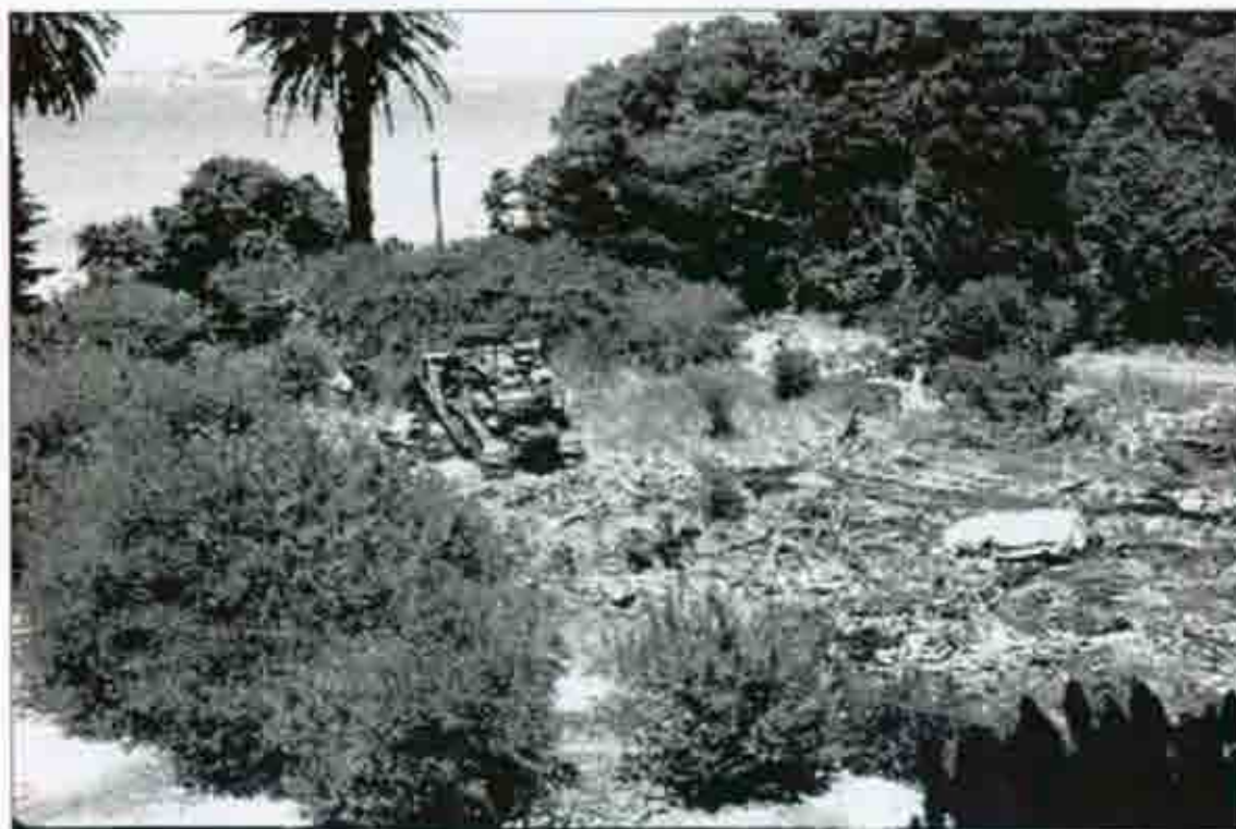
Figure 6.4. Removal of the North Garrison structures on the footprint of the former Administration Building, c.1973 (CDPR Archives).
