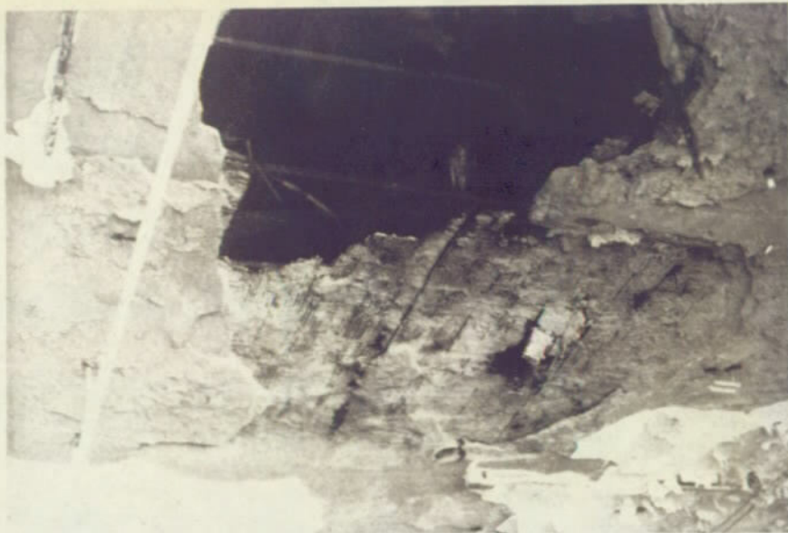
Extreme deterioration of ceiling fabric found in West Hangar Lean-To January 1979
