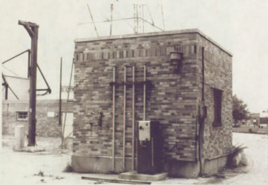
North Elevation - Missing downspout - crack at west lintel level - crack at east lintel extends around corner and up at north elevation. Note loading post at left, lower part of beacon tower behind. October 1978
