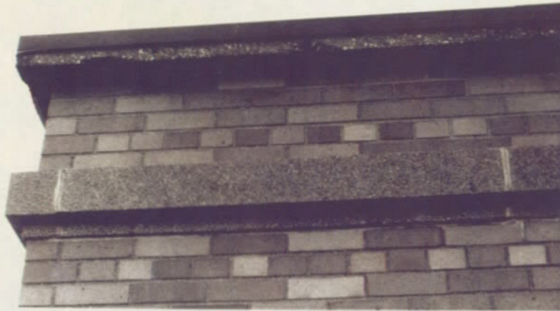
Roof of later wing - Note spalled concrete and exposed steel reinforcement.
