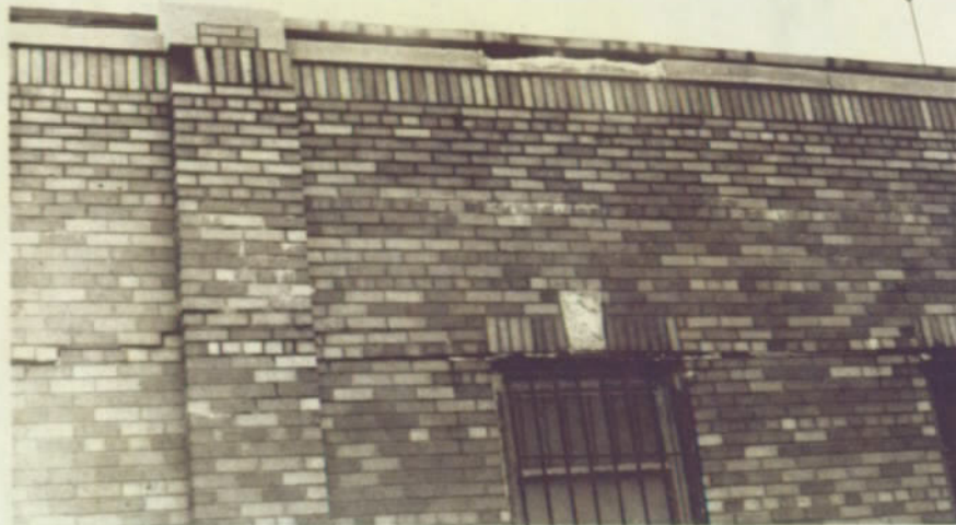
Upper wall at west elevation - note separation along lintel lines and extremely deteriorated mortar. April 1979
