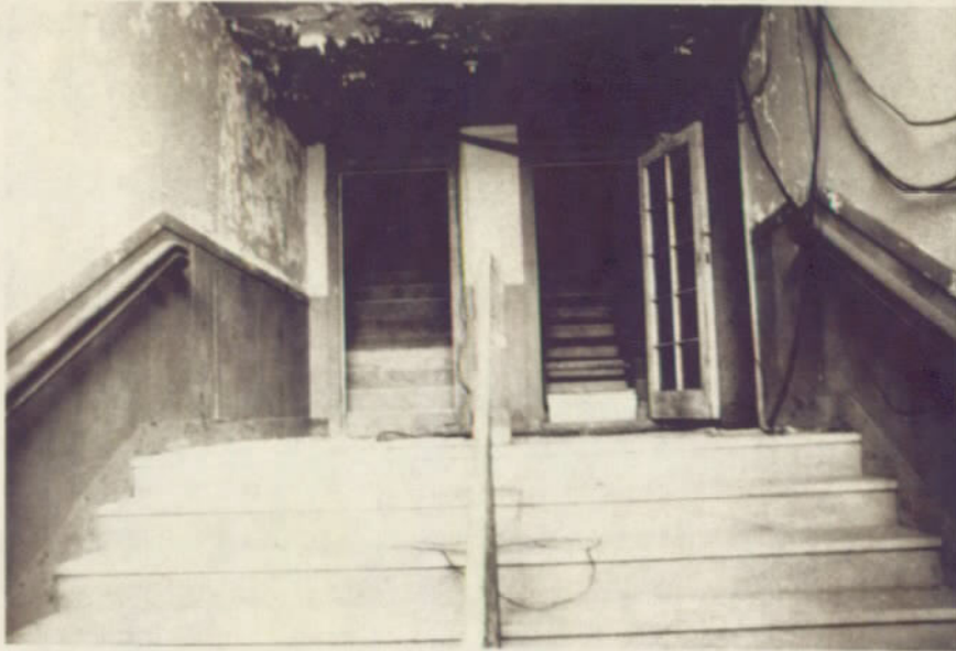
Entry out of WPA Tunnel into Administration Building. Stairs, once leading up to the first floor, have been sealed at their heads to allow for a first floor hallway across that area. Access to the basement is still possible via the barely discernible opening to the right of the stair openings. April 1979.
