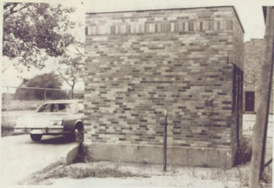
South Elevation - Note crack from lintel expansion at east extending around corner to south side. October 1978
