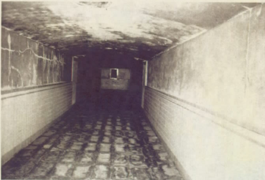
WPA Tunnel - Old wall openings have been sealed with concrete, and no documentation as to what was behind them was found. April 1979.
