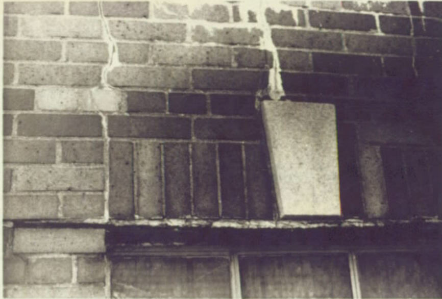
Typical window head condition note rusting, expanding lintel January 1979
