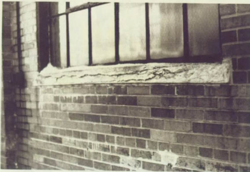
Sill condition - cast stone extremely deteriorated January 1979
