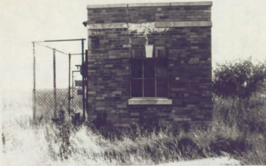
North elevation - structure is cracked both vertically and horizontally. October 1978
