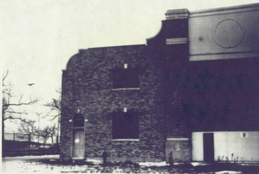
West Hangar Leanto - South elevation note loose and missing bricks at the parapet January 1979
