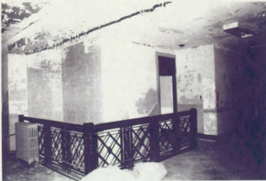
Second floor iron stair railing. Plaster walls are scored to imitate caen stone and wainscoting is buff-colored marble.
