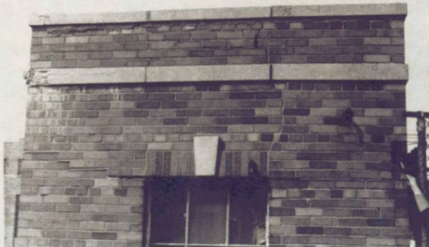
South elevation - vertical separation continues parallel to that at north. Horizontal separation continuous along lintel heights. October 1978
