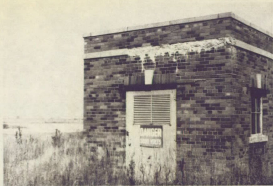
West elevation - note cast iron trim deterioration and bulge at lintel. October 1978
