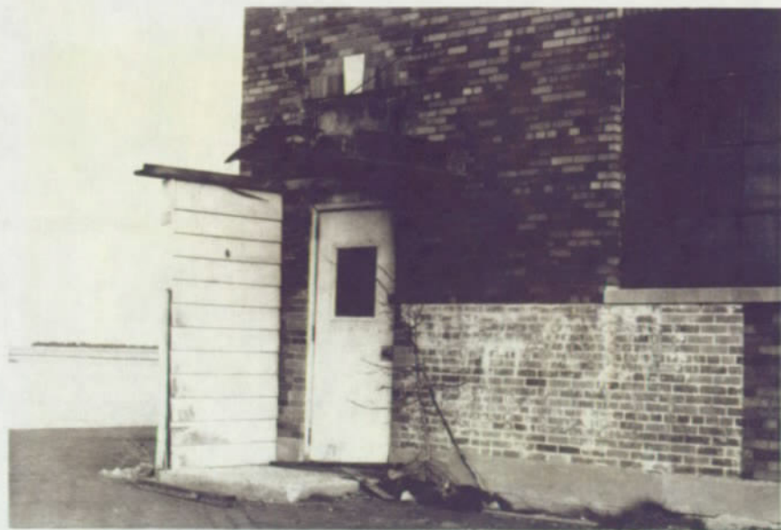
East Hangar Leanto - north door - arch above has been flattened and opening sealed , April 1979
