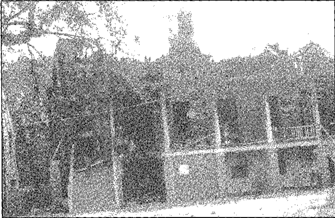
HS-1 (North elevation). Heavy fire damage destroyed the third level and exposed original timber and frame construction. Note: lower left is the original stone wall separating HS-1 and HS-2. May 1967.
