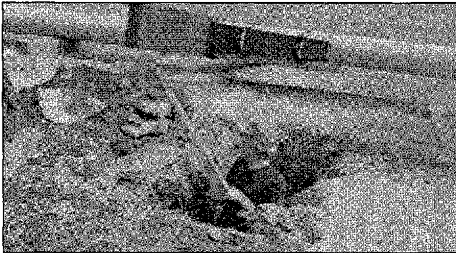
HS-16, Flagpole. Excavating foundation for subsurface flagpole base (Southwest elevation). Background: Assembled flagpole. September 1981.
