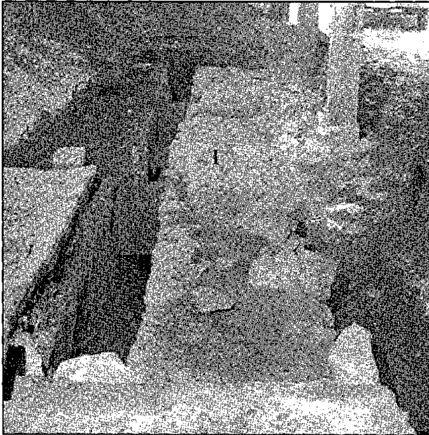
HS-8, Sept. 16, 1970: East side of the interior of the Post Hospital, looking north toward the Parade Ground. View of excavated east chimney foundation.
