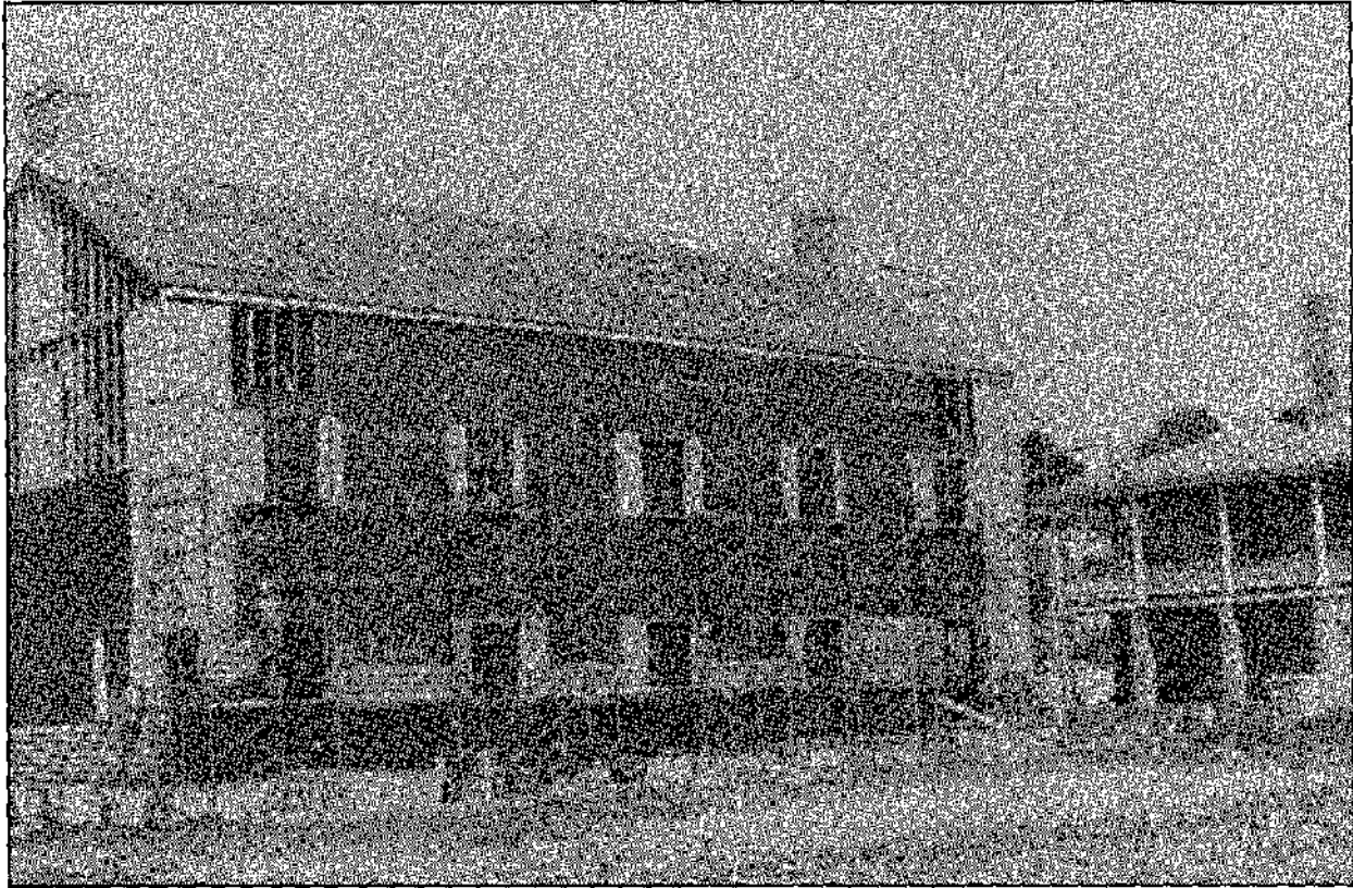
HS-7: Infantry Barracks; reconstruction in progress. Rear view (South elevation). HS-8, restored Post Hospital/Visitor Center (right). 1976.
