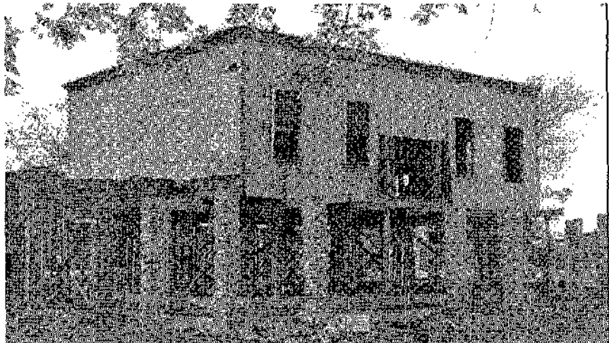
HS-8, completed stone porch pillars with a few new porch framing timbers in place. Carroll Plaza view (Northeast elevation). 1972.
