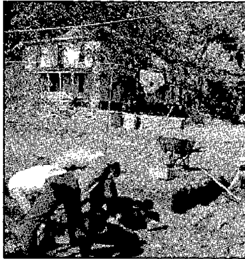
HS-22, September-October 1968: West view. Includes the northwest perimeter of the excavation with a full front and the east side of HS-12 before restoration.
