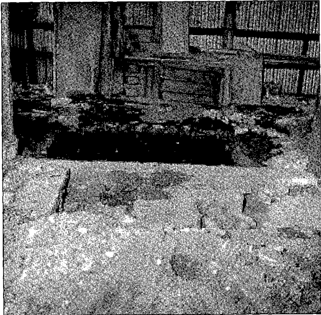
HS-8, Sept. 16, 1970: West side of the ground level of the Post Hospital looking north toward the Parade Ground. Majority of the west stone chimney foundation is visible.
