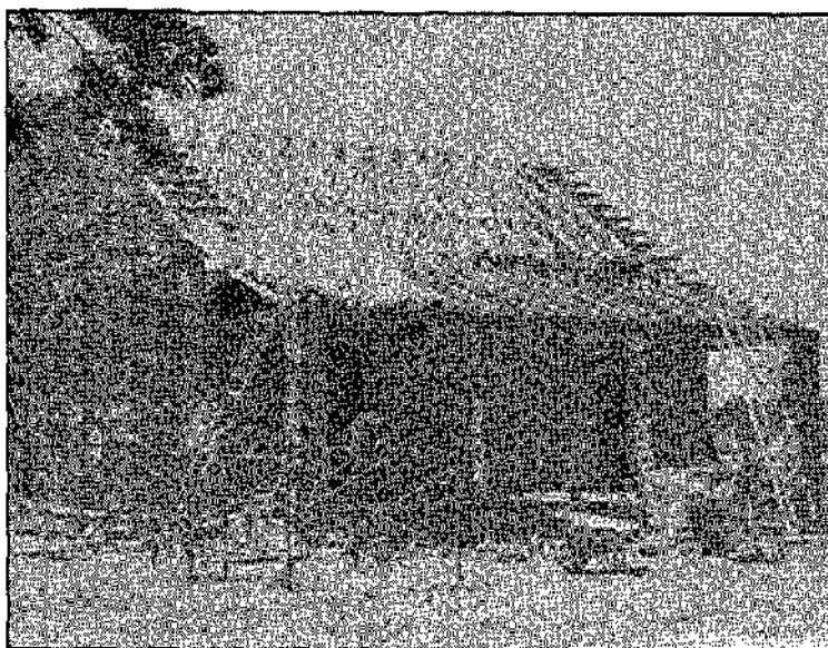
HS-9: Post Guardhouse reconstruction, installing porch roof rafters (Northeast elevation). View from Carroll Plaza. May 1975.
