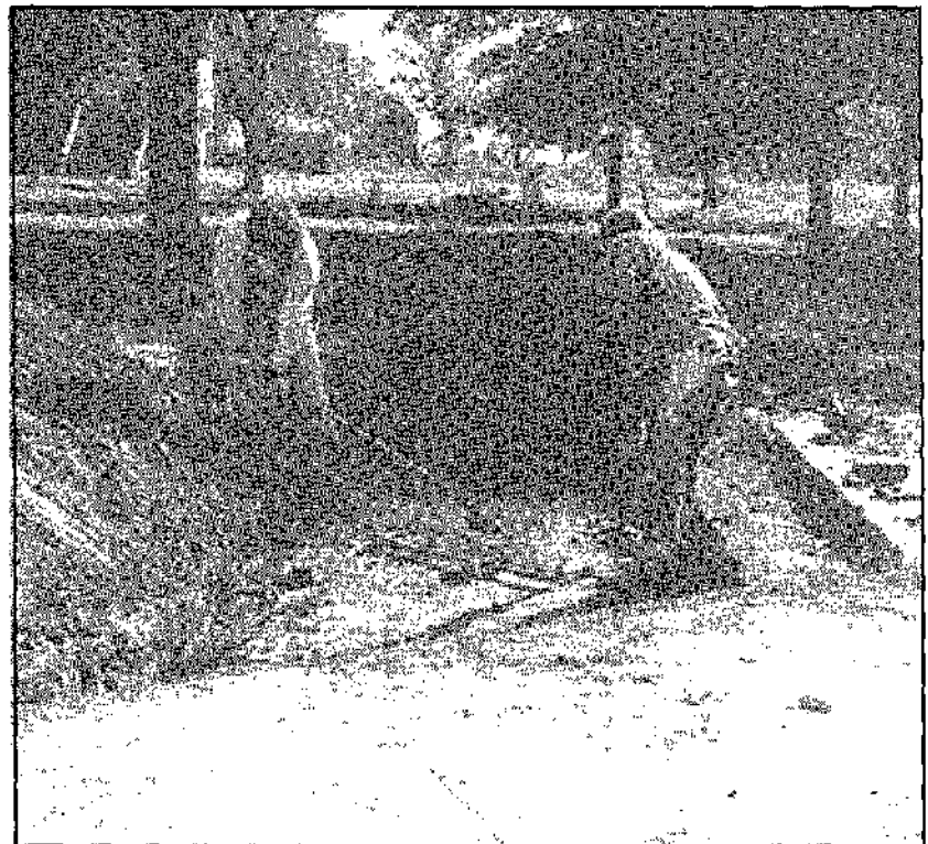
HS-15 (Well Canopy), April-July 1972: North view. Includes the west side of the octagonal-shaped structure. Buildings in the background, from left to right, include the east exterior staircase of HS-2, HS-36 (small stone out-building) and HS-19 (Lunette Blair), showing the south entrance through the earthworks.
