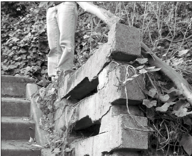
Figure 5.1.4: Concrete Slope Stabilization Cribbing. Requires further evaluation. 12/02 - OCLP.
