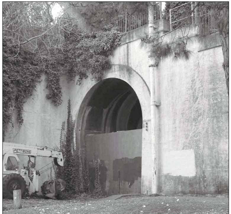
Figure 5.2.9: East Portal - Railroad Tunnel. This tunnel portal was built by the California State Board of Harbor Commissioners as part of the "Belt-Line" railroad serving the San Francisco waterfront c.1914. Contributing. 12/02 - OCLP.
