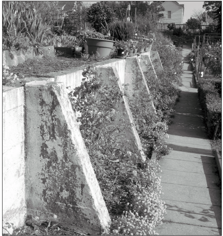
Figure 5.4.12: Foundation Remnant of Barracks, (FM - 256). Original building was constructed c1905-07 and removed between 1969 and 1972. Foundation is currently found on the northern edge of the Community Garden. Contributing. 12/02 - OCLP.
