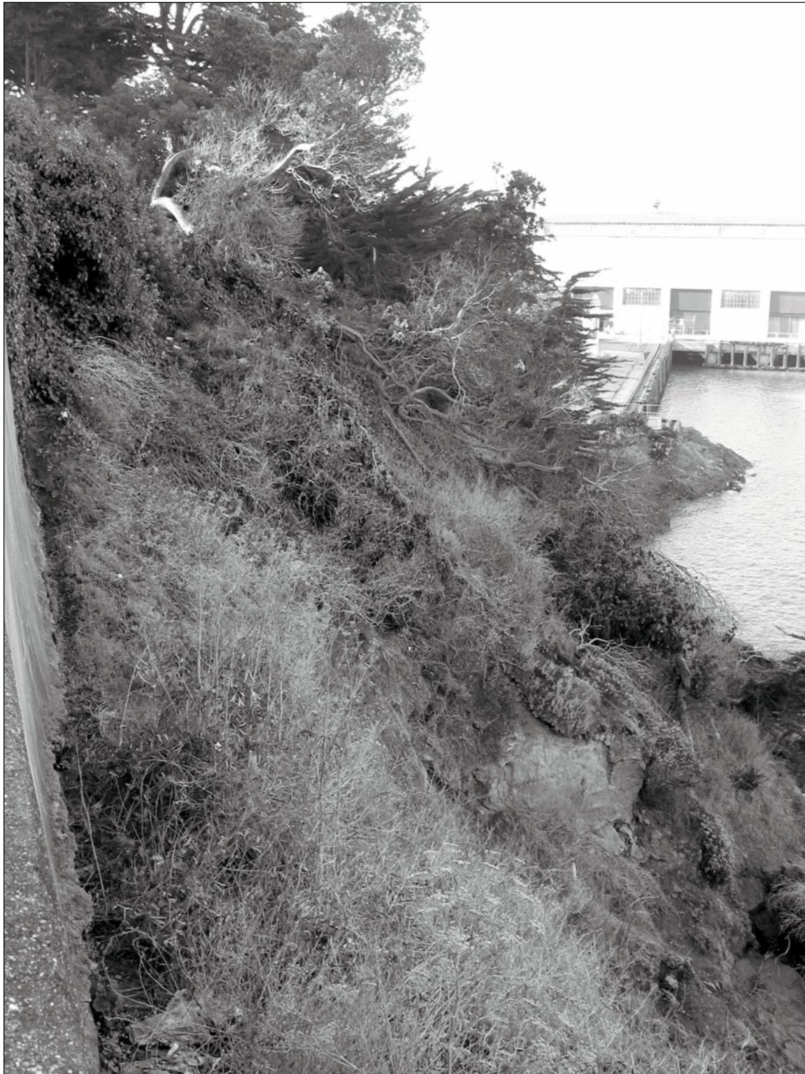
Figure 5.6.2: This area of Fort Mason's coastline represents a small area of unaltered coastal habitat within the city of San Francisco. Contributing. 12/02 - OCLP.
