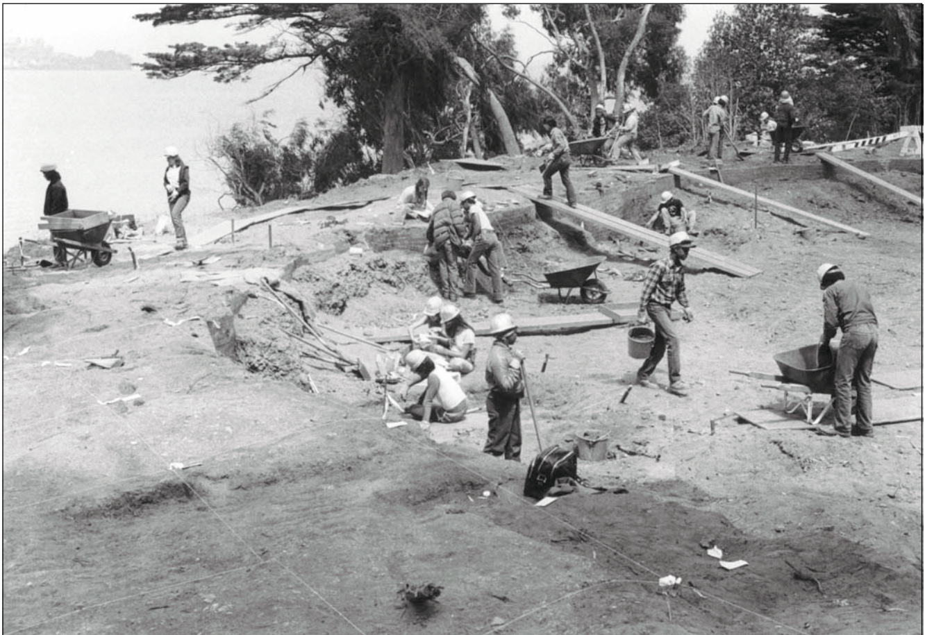
Figure 2.7.9: The earthen Civil War fortifications on the northern escarpment of Fort Mason were excavated during 1982 and 1983 and later restored. Views from this prospect remained open as late as the 1950's, after which vegetation was allowed to grow unimpeded. NPS, GGNRA, files of Park Historian.
