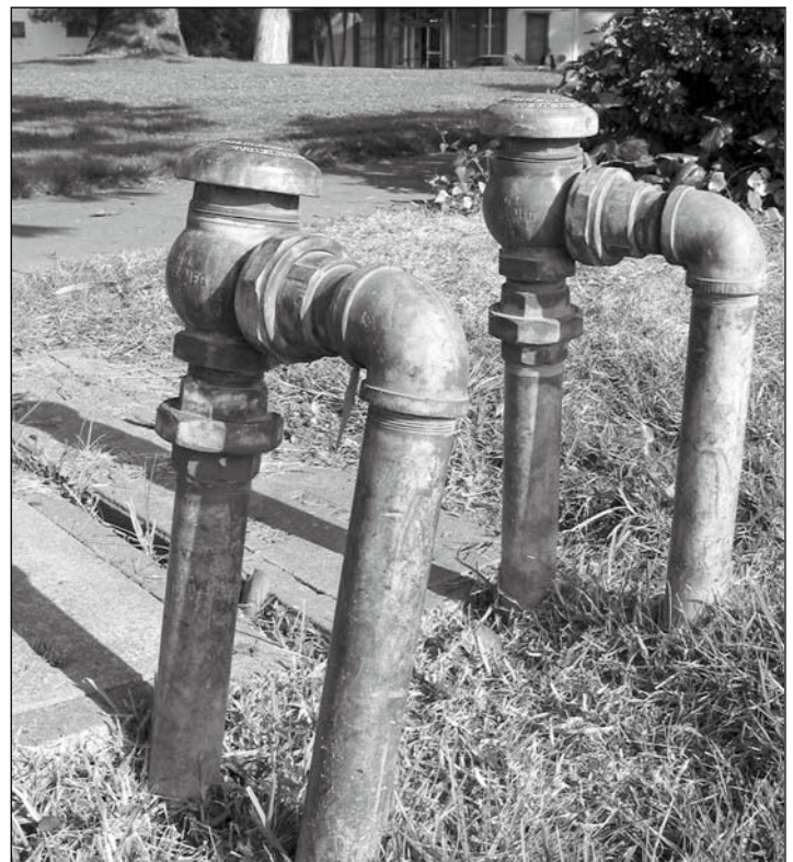
Figure 5.1.10: Irrigation System and Above Ground Fittings. While the subsurface irrigation system plays a critical role in maintaining the character of the Fort Mason landscape, the above ground expression of the system does not contribute. 12/02 - OCLP.
