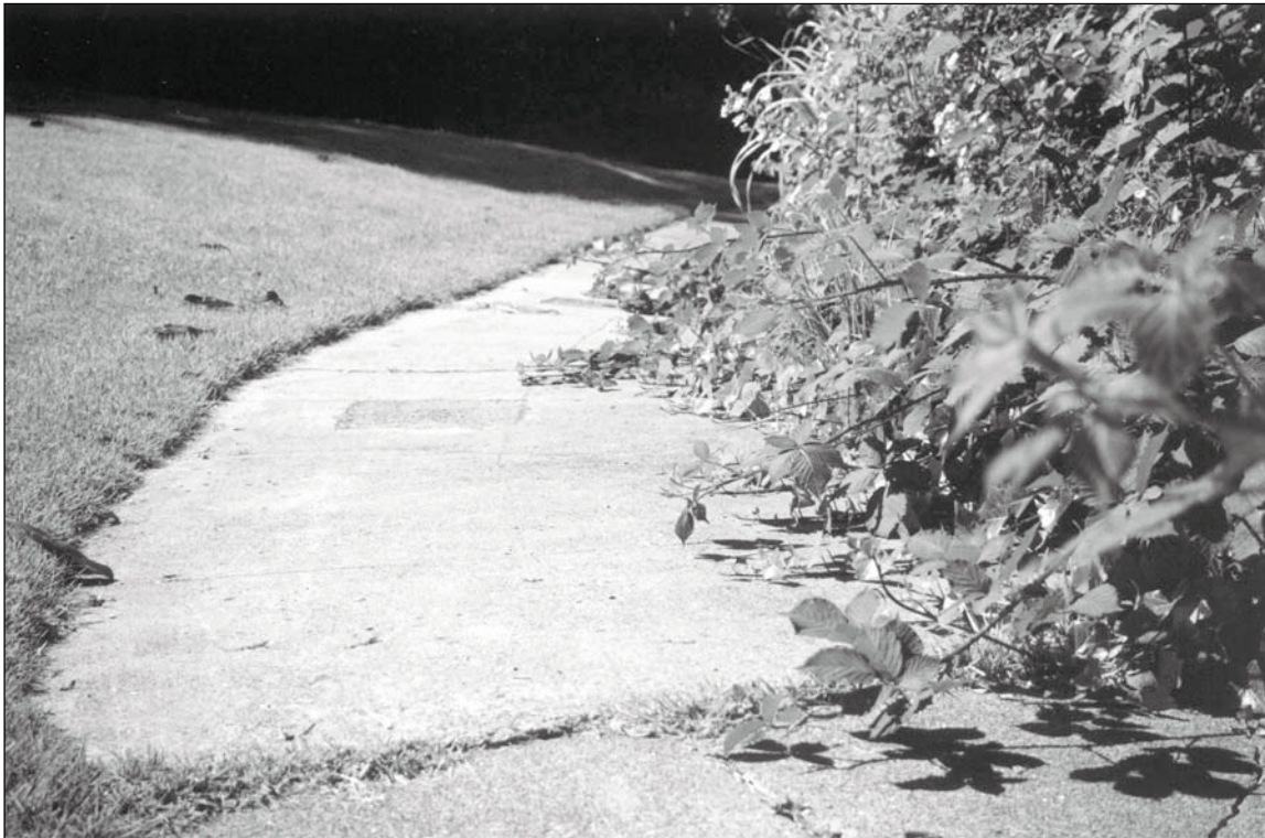
Figure 5.2.6: System of Pedestrian Paths and Stairs. The pathway system is almost entirely paved with concrete - having widths between 30" and 42." As shown above, even the best maintained segments of this pathway system require attention. Contributing. 12/02 - OCLP.
