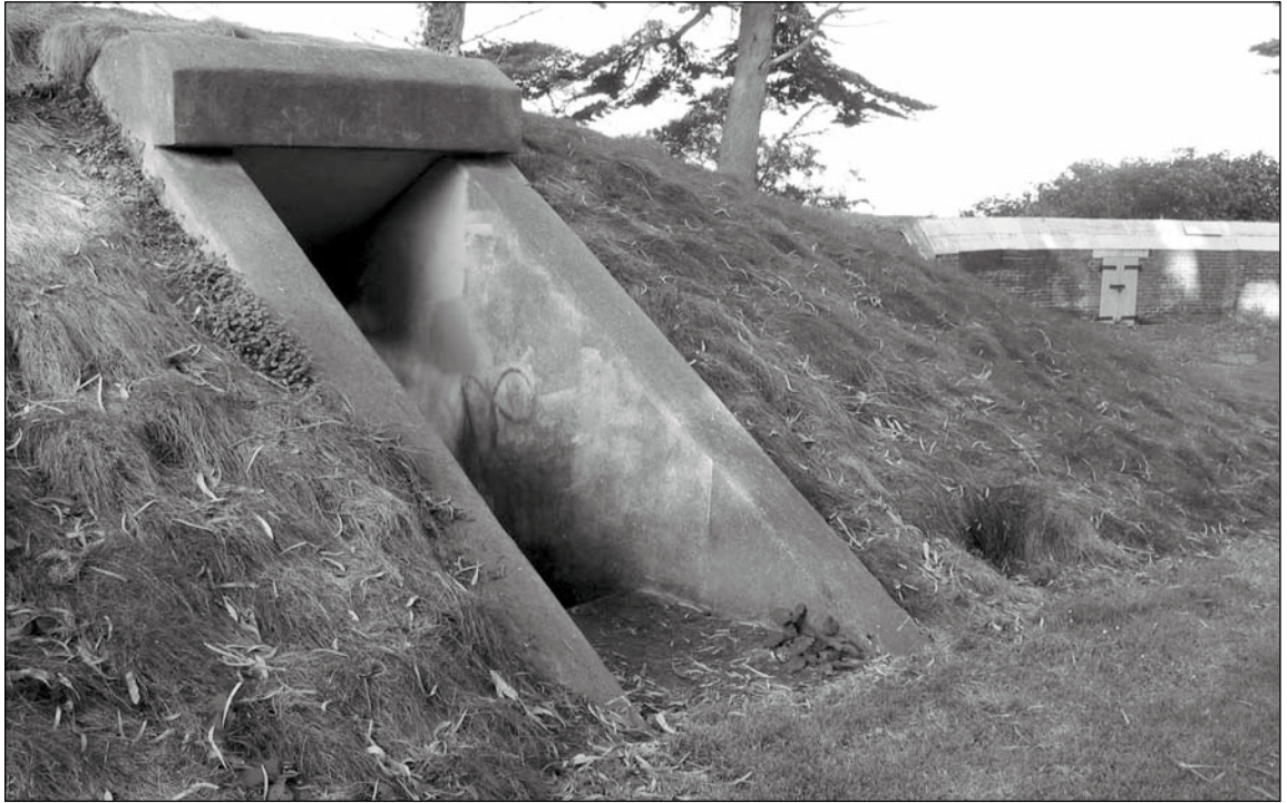
Figure 5.3.8: MLR Concrete Magazine, (FM - 250). This magazine was constructed c1898-1900, and was likely a replacement for a deteriorated earth-covered timber magazine at the same location. Contributing. 12/02 - OCLP.
