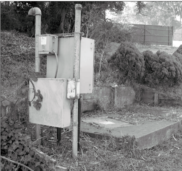
Figure 5.1.16: Utility Service Cabinets and Panels. The underground electrical and telecommunications system is a significant aspect of the character of Fort Mason. The physical above-ground expression of this system in the form of service panels and cabinets is not significant. Non-contributing. 12/02 - OCLP.
