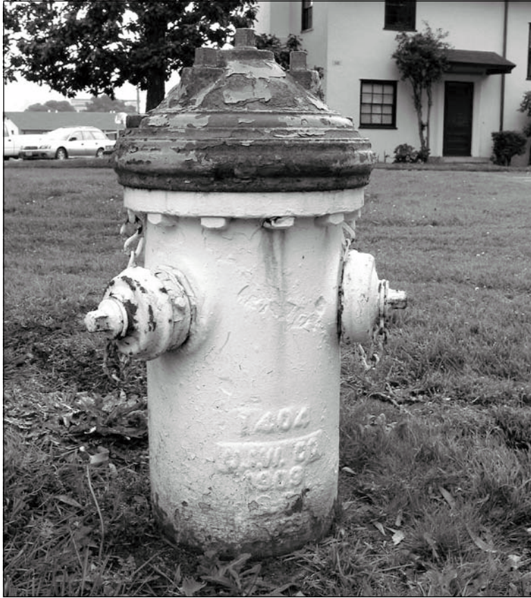
Figure 3.1.21: Small-scale features. The fire hydrant shown above is part of a high-pressure emergency backup system designed and installed following the catastrophe of 1906. The year 1909 is cast into the body of the hydrant. In the event of an emergency, it is supplied with salt water from the pumphouse at the foot of Van Ness Avenue. 12/02 - OCLP.
