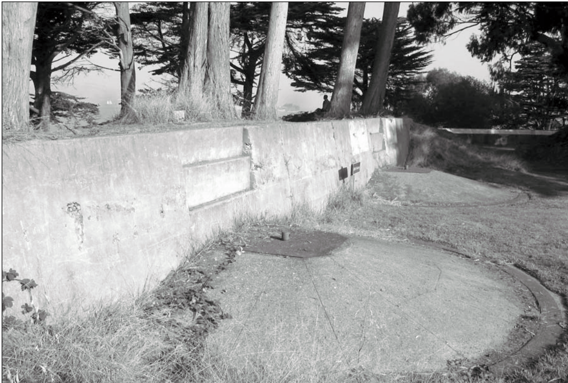
Figure 5.3.10: MLR Concrete Gun Platform, (FM - 329A). These two gun emplacements were begun as an emergency measure during the Spanish-American War. Contributing. 12/02 - OCLP.
