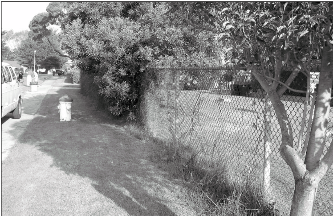
Figure 5.2.18: Chain-link fencing at Franklin Street Frontage. The date of the replacement of the original wooden fencing on this site with wire-fencing is uncertain, but is likely to have occurred prior to WWII. Feature requires further evaluation. 12/02 - OCLP.
