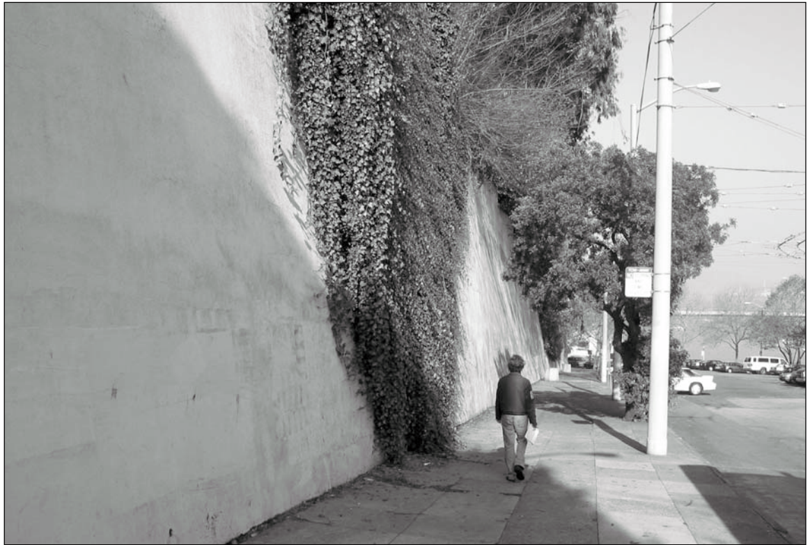
Figure 5.2.12: Van Ness Avenue Retaining Wall. This wall was built in two sections. The southern section appeared c.1900, associated with the relocation of the post entrance to the corner of Van Ness Avenue and Bay Street. The northern section was built c.1910, associated with the extension of Van Ness Avenue and the construction of the city's emergency pumping station. Contributing. 12/02 - OCLP.
