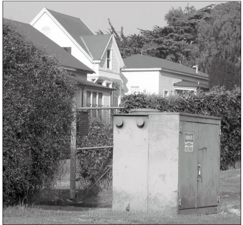
Figure 5.1.17: Utility Service Cabinets and Panels. Non-contributing. 12/02 - OCLP.
