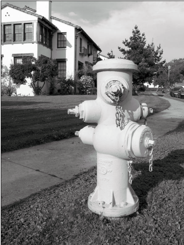
Figure 5.1.7: The inventory of fire hydrants, other than the Emergency High Pressure Hydrants, requires further evaluation as to their historic status. 12/02 - OCLP.
