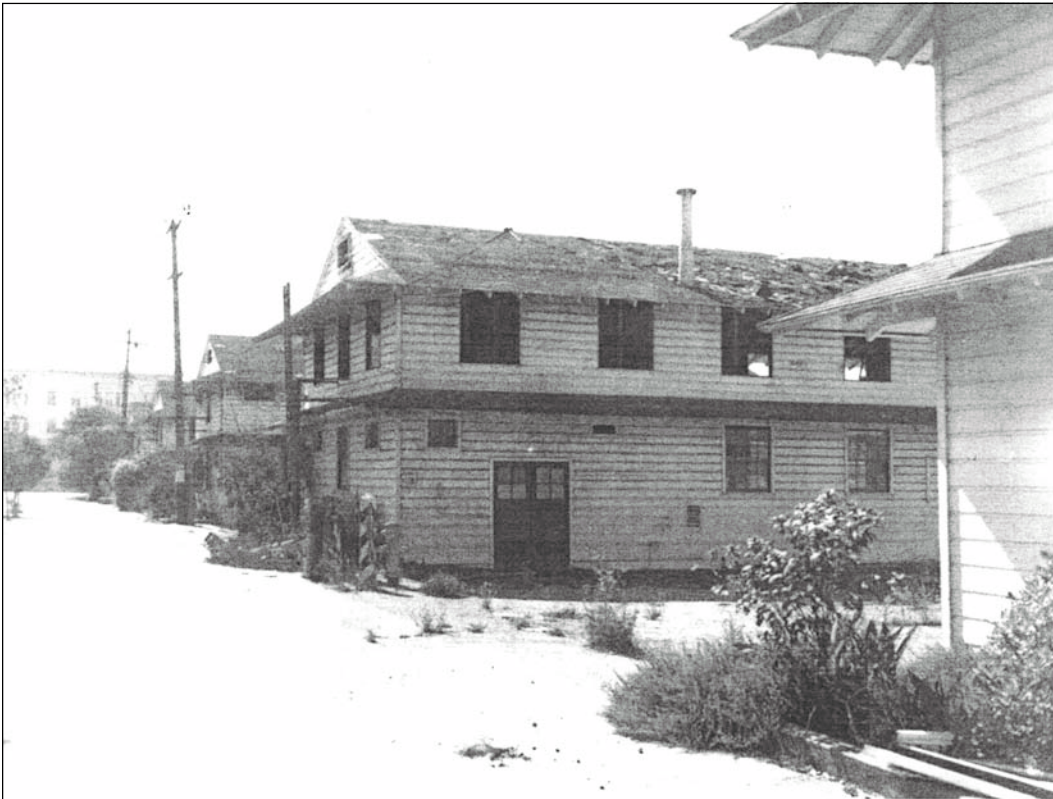
Figure 2.6.12: Many of the temporary buildings constructed at Fort Mason during the 1940's were in poor condition prior to the NPS acquisition of the property. The NPS was in the process of salvaging these buildings when this photograph was taken. Photo by John Martini, c.1977. NPS,GGNRA Archives, Interpretation Photograph Collection, GOGA-2316.
