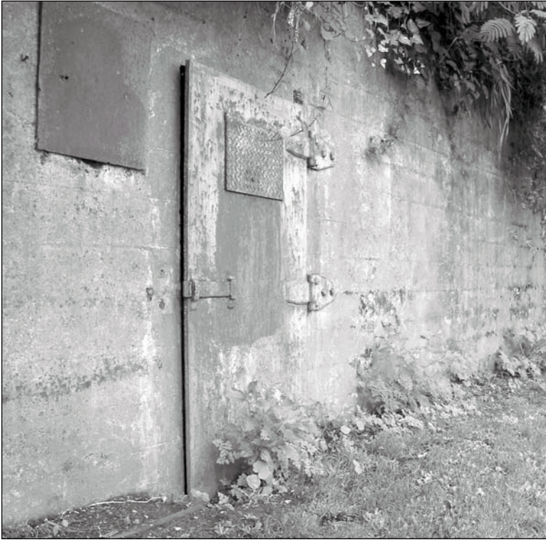
Figure 5.2.10: Mine Casemate and Mine Casemate Retaining Wall. Apparatus within this subterranean room controlled harbor mines between 1891 and 1945. The retaining wall was built c.1910 contemporary with the construction of the adjacent emergency pumping station. Contributing. 12/02 - OCLP.
