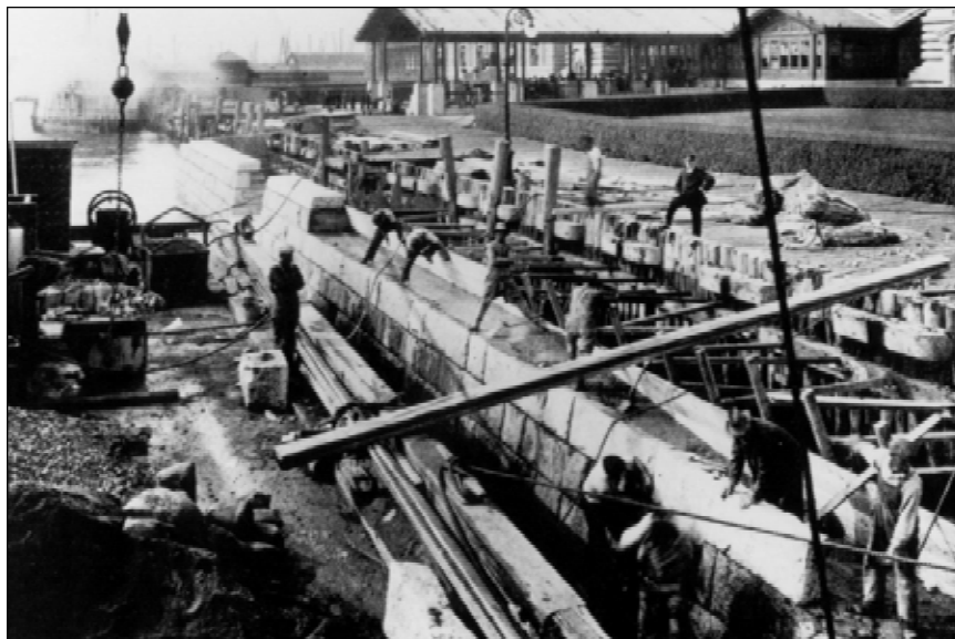
Figure 4.17 In 1913 construction began on the new concrete and granite seawall on Island One. This image of construction on Contract #1 shows how the new seawall was placed outside the existing crib bulkhead, reducing the width of the ferry basin by about thirty feet when the north and south basin seawalls were completed. Circa 1913. (STLI Library, 26.7, #16)
