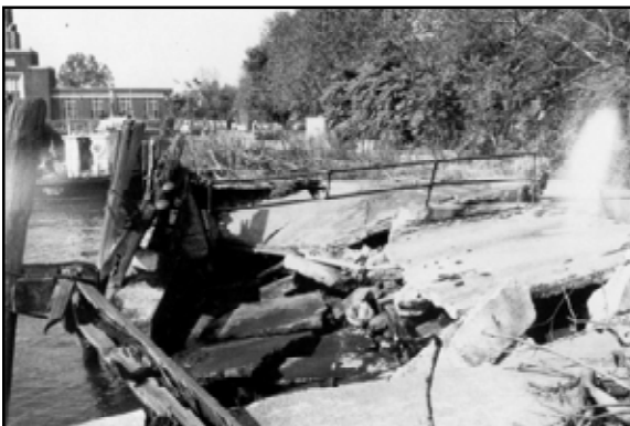
Figure 6.5 During the early 1970s, much of the island remained in a derelict state, as illustrated by this deteriorated section of seawall and walkway along the north side of the ferry basin on Island One. October 1973. (STLI Library, 26.7, #2)
