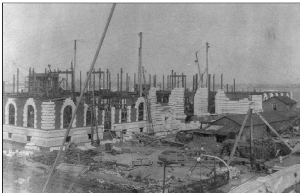
Figure 3.2 Construction of the main immigration building. Notice the wooden fence remaining from the earlier building in the foreground. June 30, 1899. (National Archives and Records Administration, RG121-BCP-37D-6)
