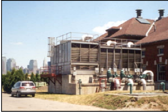
Figure 6.25 A service area containing fuel tanks and HVAC units is located north of the powerhouse on Island One. August 2002. (Photo by author)
