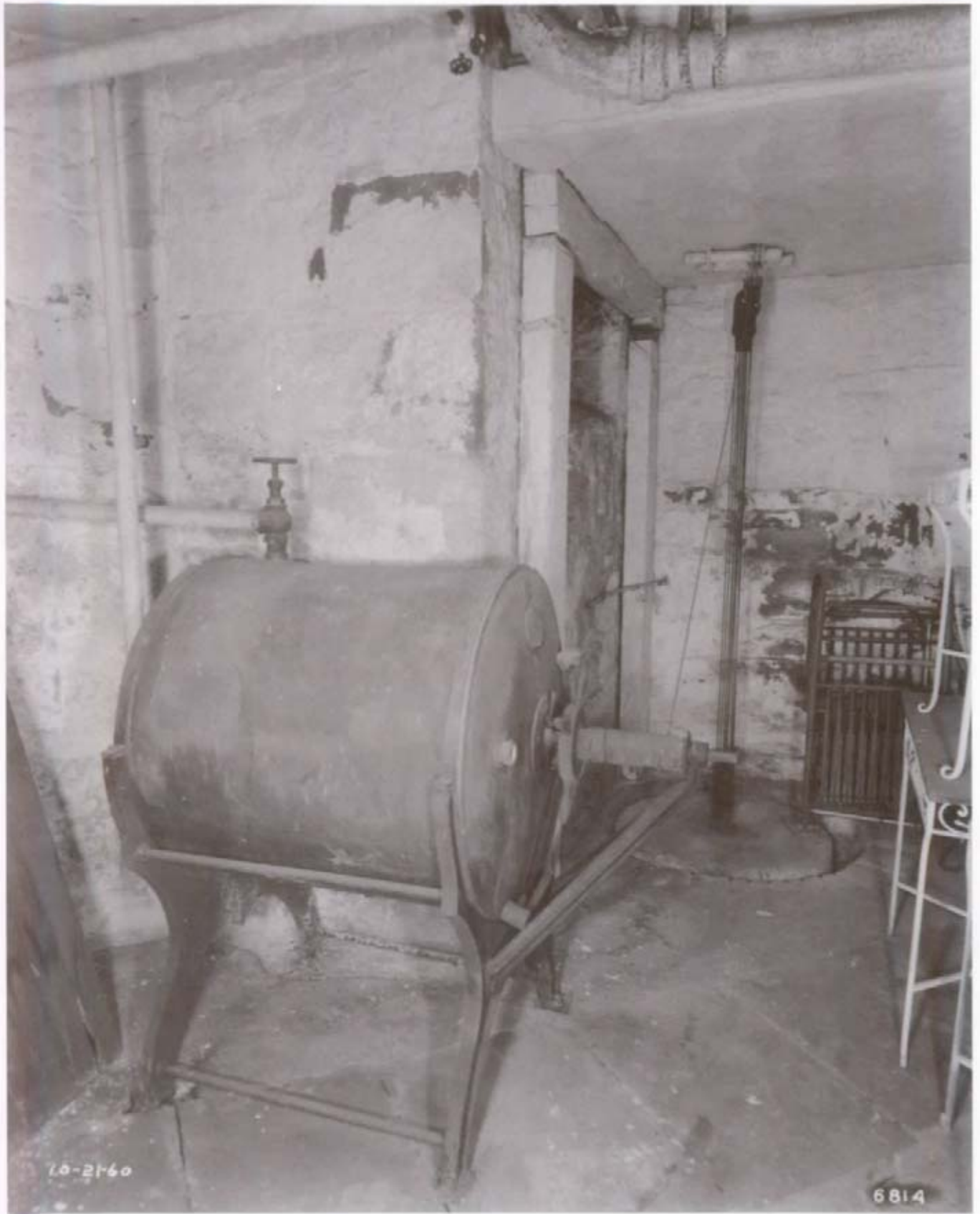
Figure 37. Room B9, northeast corner, showing the obsolete Springfield Gas Machine, 1960.
