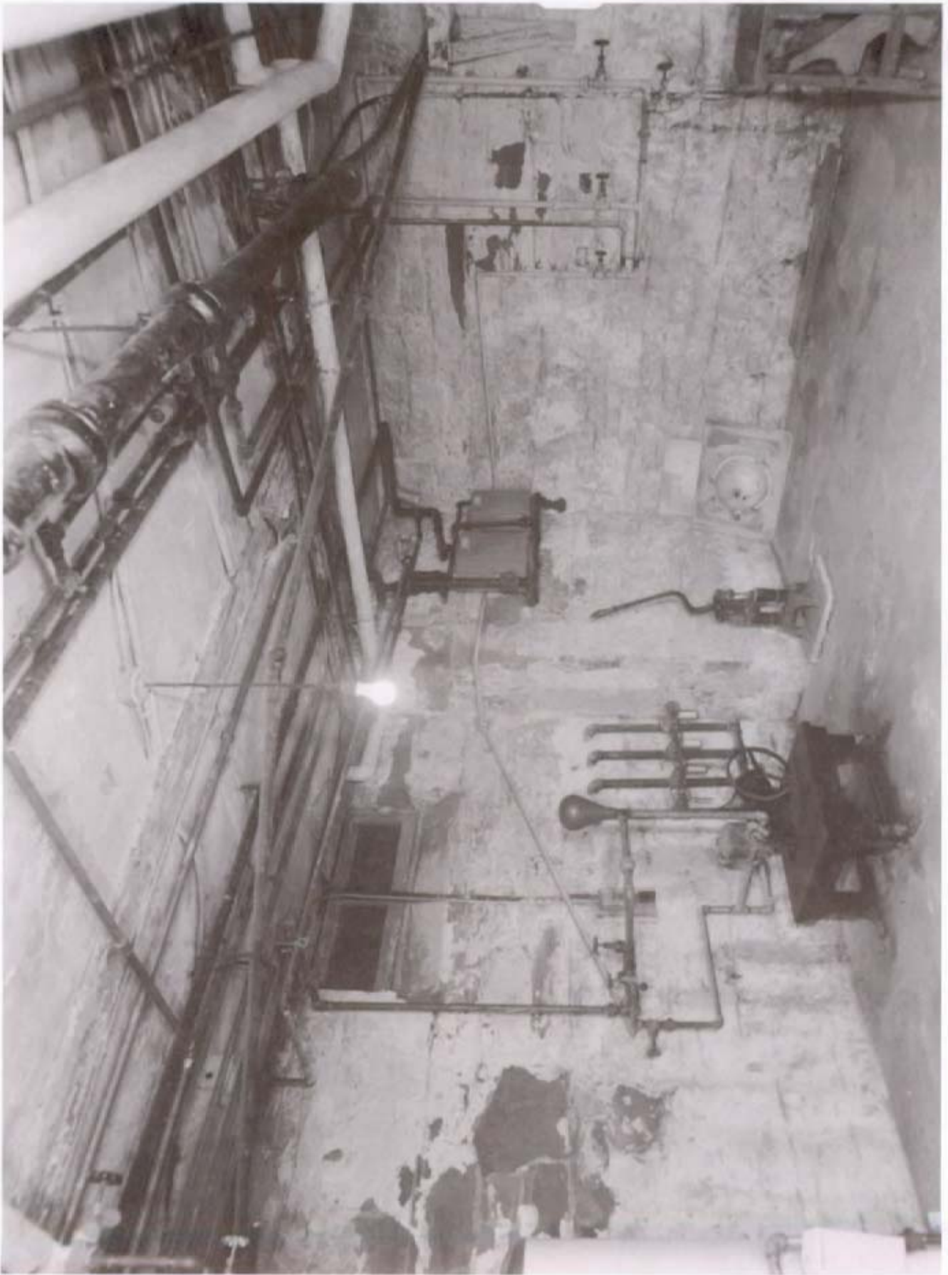
Figure 39. Pump Room (Room B14), northwest corner, showing the cistern valves and water pumps, 1960.
