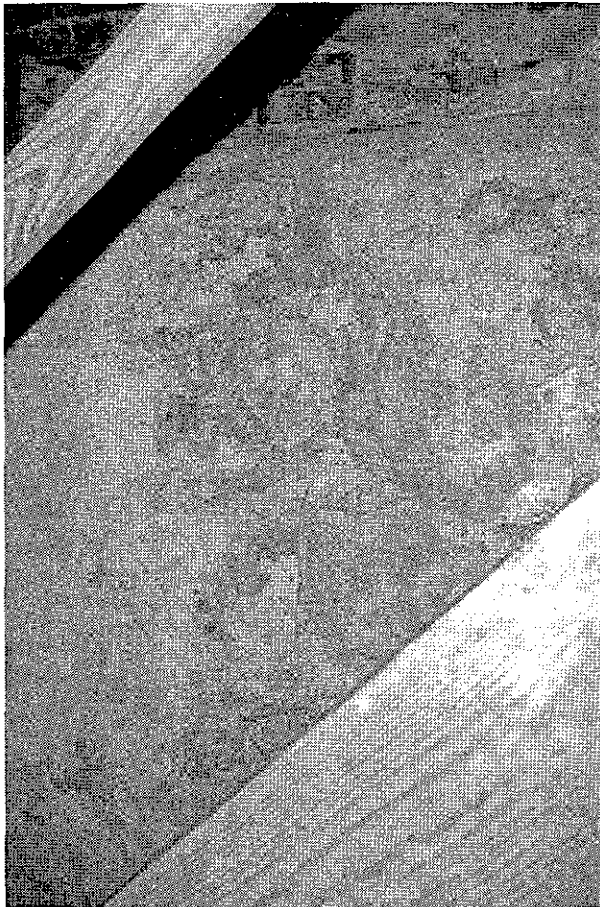
Figure 1 View of the cracked and missing parging of the south foundation wall at the stair, 1996 (Fitzpatrick Structural Engineering).
