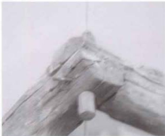
Figure 28 Detail of typical ridge connection in original roof, from partial rafters now in CARI Collection. (NPS-SERO-CRS, 2001)
