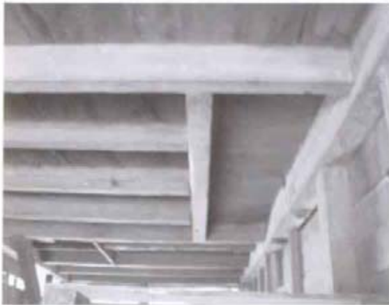
Figure 22 Ceiling in "lint room," showing framed opening for ginned cotton from first or second generation gin at second floor level. (NPS-SERO-CRS, 2001)
