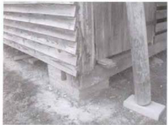
Figure 18 View of northeast corner of barn, showing brick pier rebuilt in 1996. (NPS-SERO-CRS, 2001)
