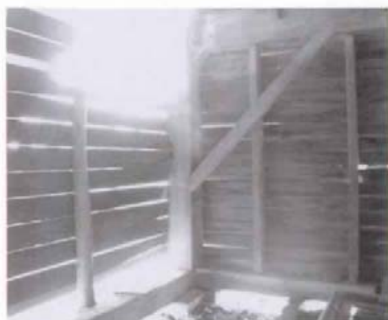
Figure 25 View of southwest corner of barn; wall at right was added in the late nineteenth or early twentieth century. (NPS-SERO-CRS, 2001)
