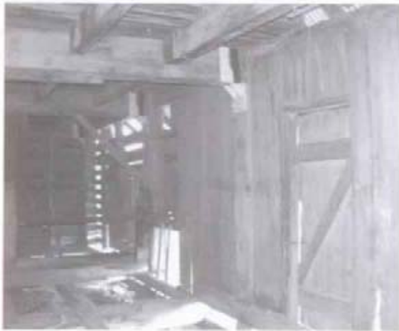
Figure 16 View southeast in machinery room, in probable location of original seed room. (NPS-SERO-CRS, 2001)
