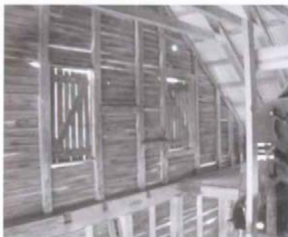
Figure 26 View to southeast showing part of east end of barn; note empty mortises for framing around missing stairway. (NPS-SERO-CRS, 2001)
