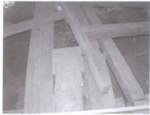
Figure 23 View of framing members in floor at east end of gin barn, with end of hewn beam visible at center, presumably from first cotton press. (NPS-SERO-CRS, 2001)
