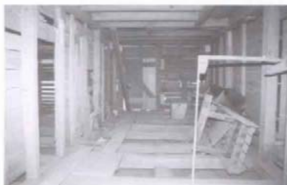
Figure 15 View north in center room, originally used as a lint room. (NPS-SERO-CRS, 2001)
