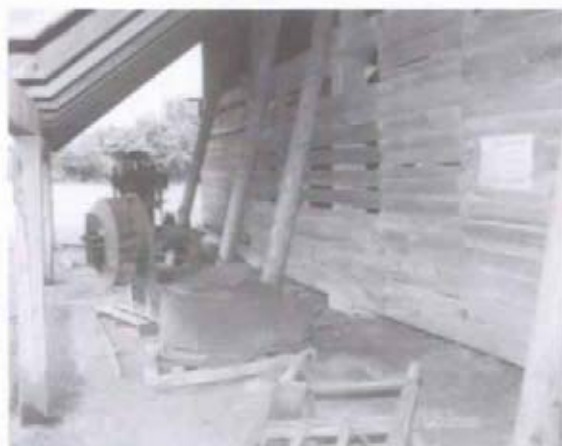
Figure 42 View west under south arcade, showing blowers and other equipment associated with c. 1900 system gin. (NPS-SERO-CRS, 2001)
