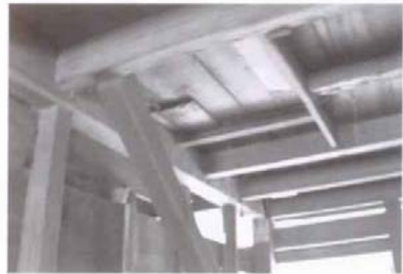
Figure 24 View of framing in lint room ceiling for cotton bale slide which was added along with new hydraulic press around 1900. (NPS-SERO-CRS, 2001)
