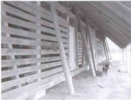
Figure 32 View of north side of building, showing typical open siding. Note that siding near center is attached to the interior face of the studs. (NPS-SERO-CRS, 2001)
