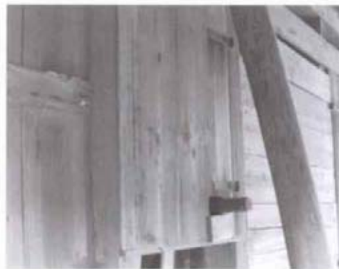
Figure 36 View of window H, which originally had sash but was closed when existing gin machinery was installed c. 1900. (NPS-SERO-CRS, 2001)
