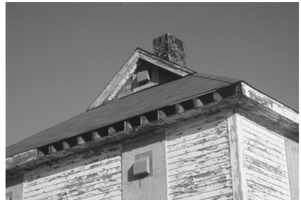
Figure C-5 Missing fascia board on the north elevation
