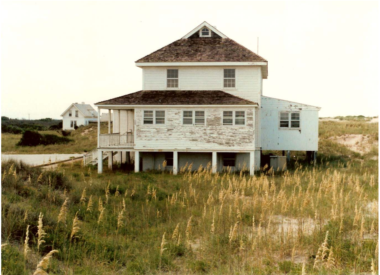
H.28 1925 Station view from the south, Dec. 1986. Shows the 1962 lean-to addition to the front to the building, and the c. 1956-62 enclosure of the south porch.
