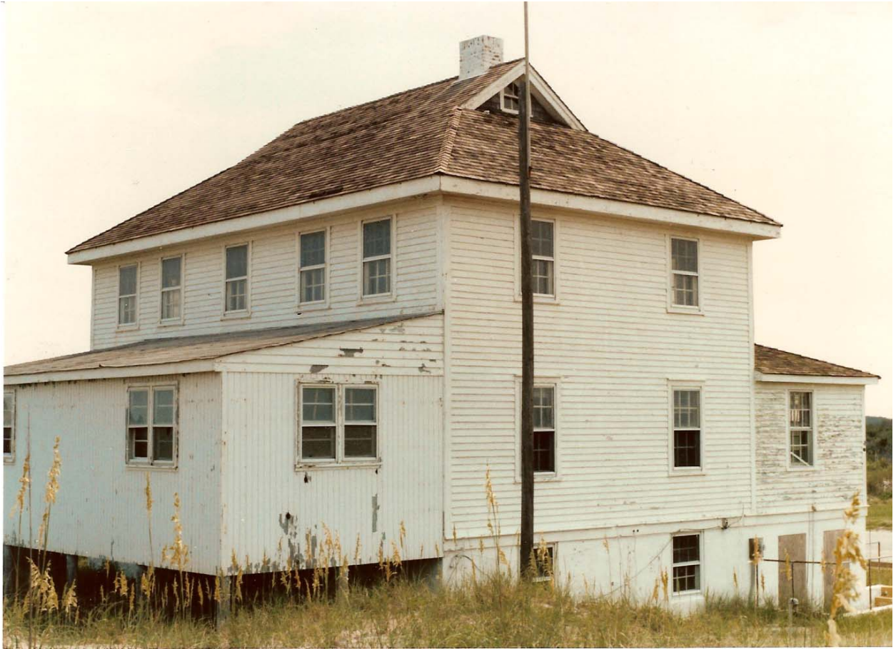
H.27 1925 Station view, Dec. 1986. Shows north and east facades, with the 1962 lean-to addition to the front to the building.
