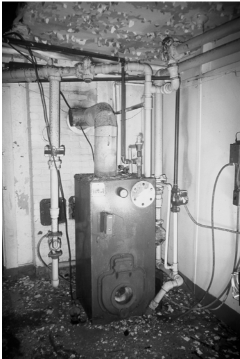
Figure C-19 Oil Boiler in Room 006
