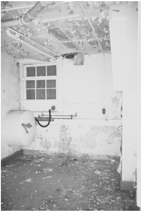
Figure C-15 Tank in Room 003
