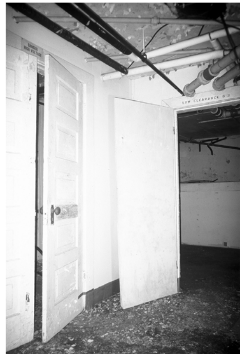
Figure C-18 Reused 1925 double doors from Room 005 (L) and shortened doorway from Room 004 with modern door (R).
