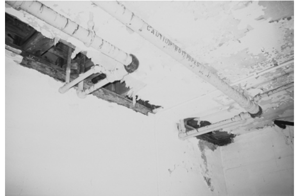
Figure C-13 Termite damage to ceiling joists and sill plate
