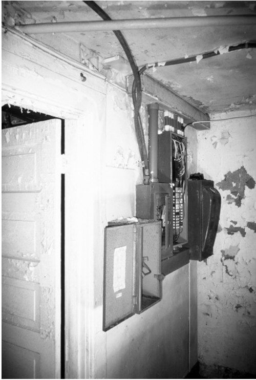
Figure C-17 Electrical Panels in Room 005
