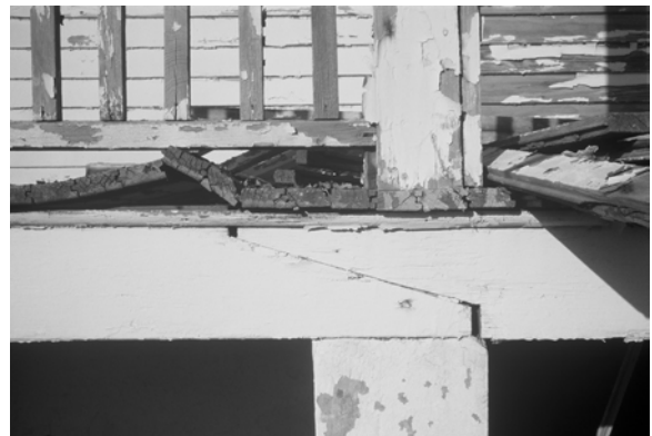
Figure C-8 Buckling porch flooring and collapsed porch railings
