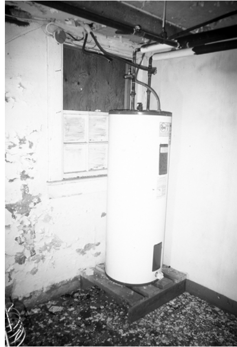
Figure C-20 Electric water heater in Room 006 • Other Features: None are present.
