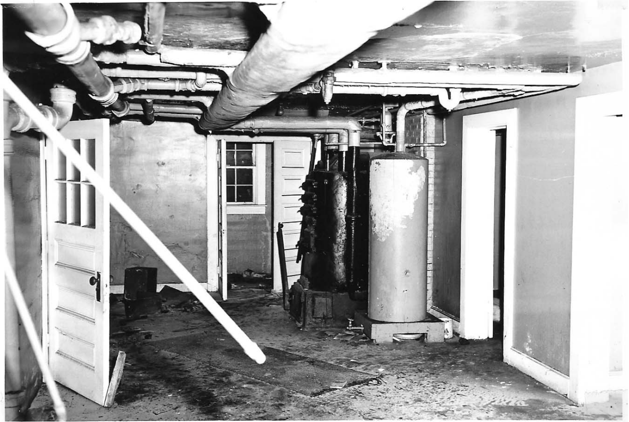
H.20 1925 Station looking north into generator room basement level, March 30, 1954 by J.C. McCabe, Photo no. 5. Label: "Basement, Bodie Island C.G. Sta."
