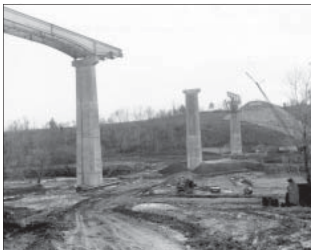
Figure 6.22. Construction of the Hales Ford Bridge during the building of Smith Mountain Lake. January 18, 1962. American Electric Power Company construction files. Roanoke, Virginia. RB .577.
