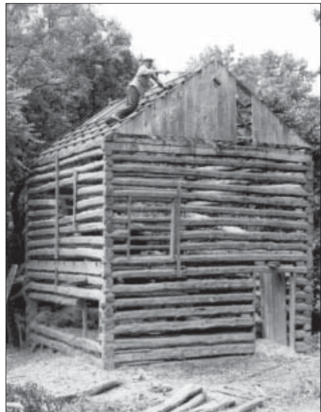
Figure 6.6. Repair of the tobacco barn. The barn contains logs that date to the Burroughs period. 1958. BOWA files.
