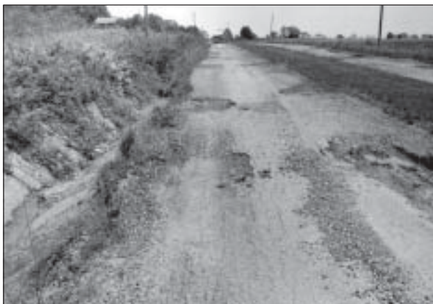
Figure 6.1. Deteriorated entry road as it appeared when the National Park Service (NPS) acquired the site. Circa 1958. BOWA files.
