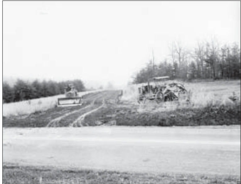
Figure 5.4. Construction of the new Birthplace Memorial driveway. Note the old entry drive along the tree line at the far right of the image. 1946. BOWA files.
