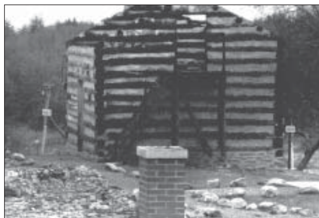
Figure 5.19. Taken immediately after the former headquarters building fire, dated posts of the "Booker T. Washington in Electrical Illumination" exhibit appear unharmed behind the damaged cabin replica. 1950. BOWA files.
