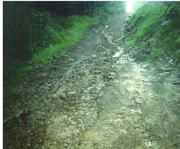
5-21 Severely eroded road – ideal conditions for broad based dips.
