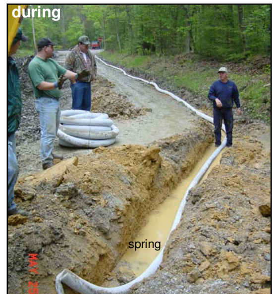
Photo 2. Pre-fabricated underdrain was used to collect subsurface water from under the road and both ditches.
