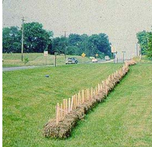
5-04 Proper bale installation prior to start of a major construction project. (Note: Bale barriers not recommended by EPA.)
