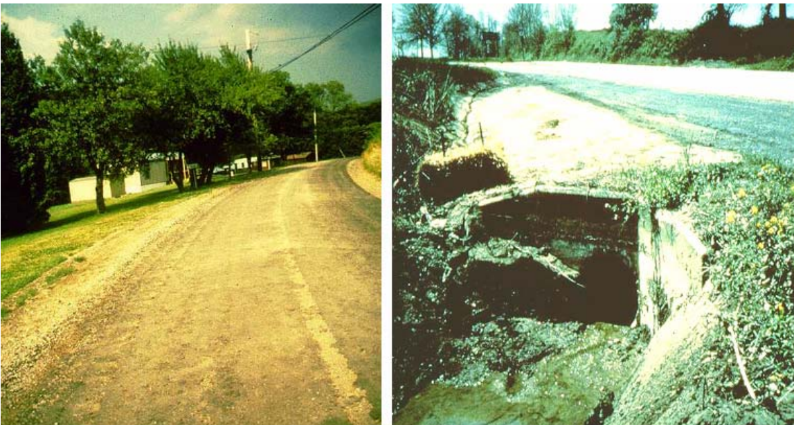
7-09 With the use of asphalt “oils,” tracking and/or run-off can become problems.
