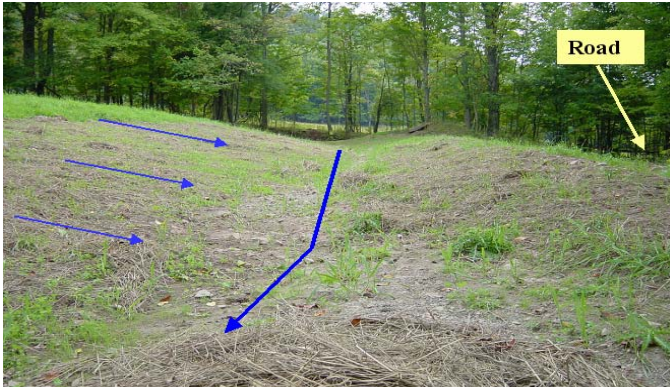
ESMP#13-02 Diversion Swale: Wider swales and gradual slopes result in more infiltration and less water volume to handle.
