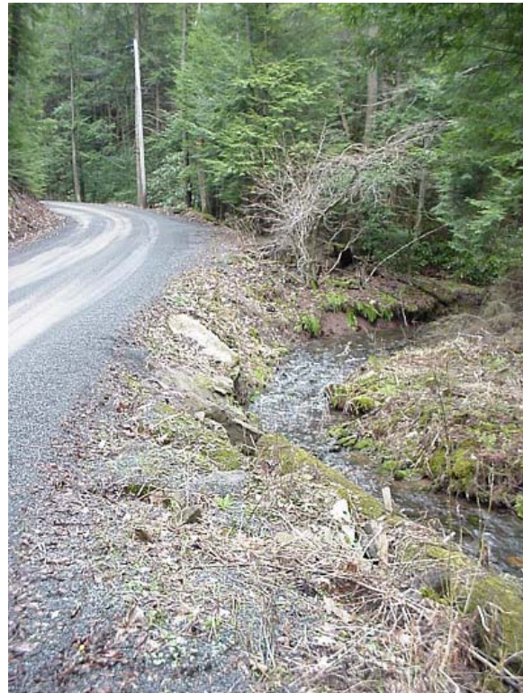
6-01 Typical roadside erosion problems.
