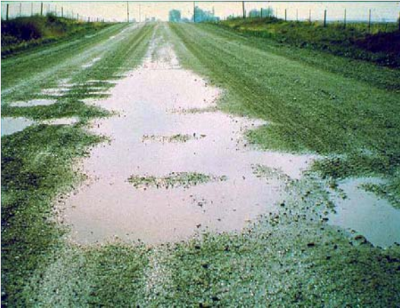
3-08 Water quickly collects when the road crown is lost.
