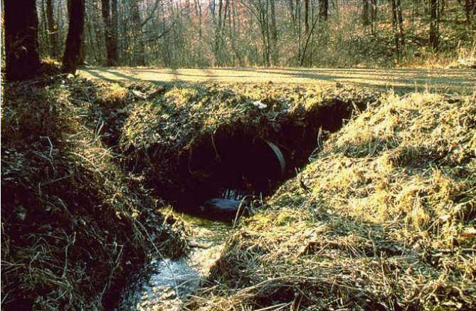
5-19 Do not outlet ditch directly to stream—use turnouts into vegetative filter strips!
