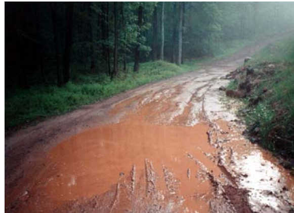
4-08 Concentrated water flows cause many familiar maintenance problems.
