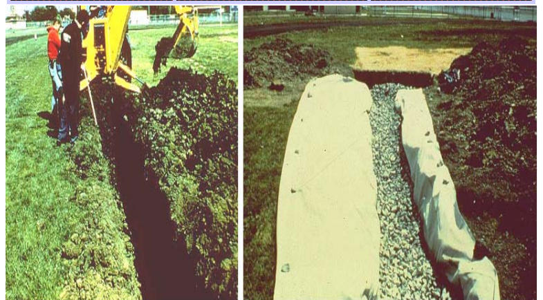
7-20 Subdrain construction - dig trench, roll out fabric, add pipe and aggregate, overlap fabric, backfill.
