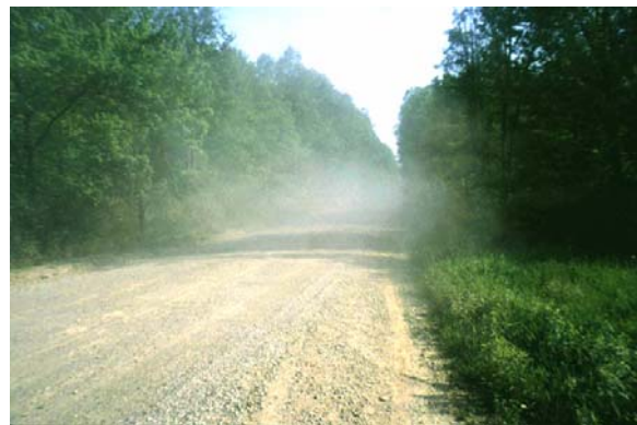
7-01 Unpaved roads are the largest source of dust pollution in the country.
