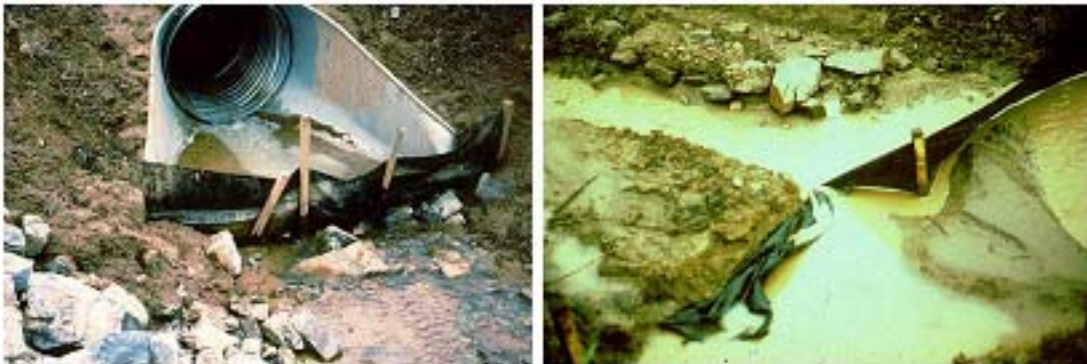
5-05 Improper silt fence installations.
