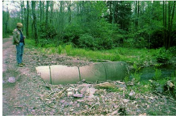
A7-01 Hell Hollow Road Demo Site: Existing site conditions prior to project.
