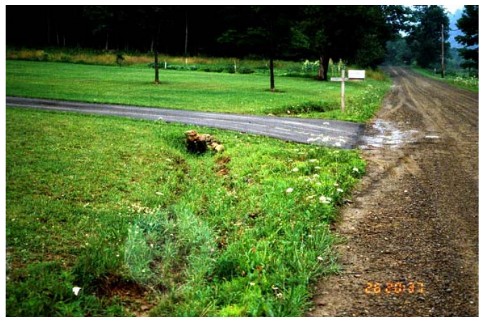
5-25 Improperly constructed driveways create recurring road maintenance problems.
