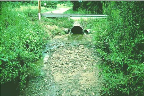
5-02 Once erosion takes place, the sediment needs to be addressed.
