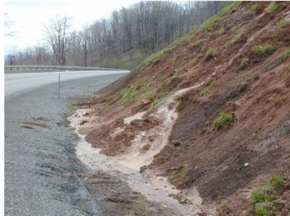
2 - 07 Flowing water picks up volume and velocity causing further erosion.
