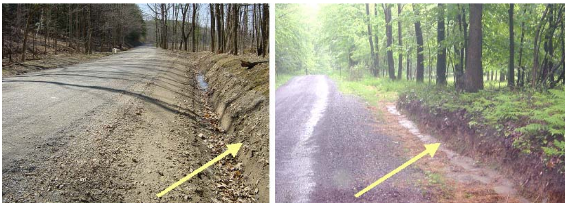
6-25 Unstable vertical bank will collapse.
