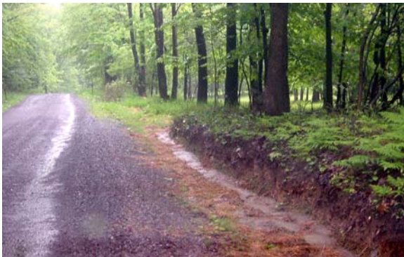
3-04 Roads interfere with natural systems, causing accelerated erosion
