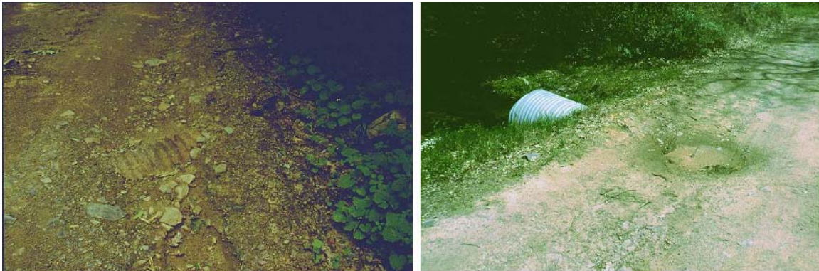
ESMP#9-01 Shallow pipe installations can cause continual road deterioration.
