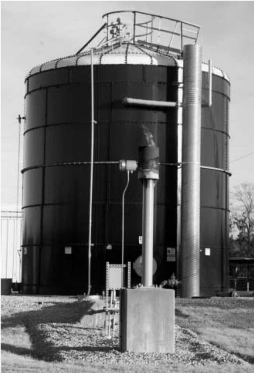
Biogas flare burns at the University of Florida's fixed-film anaerobic digester.
