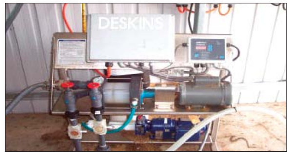
Polymer Preparation Unit
