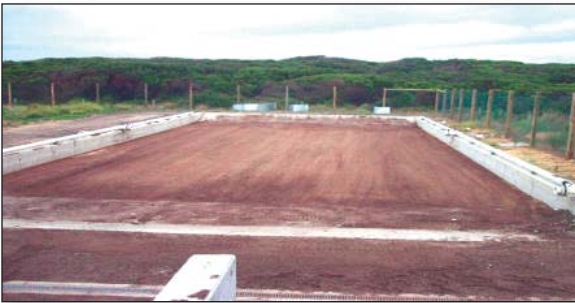
Deskins Quick Dry Filter Bed
