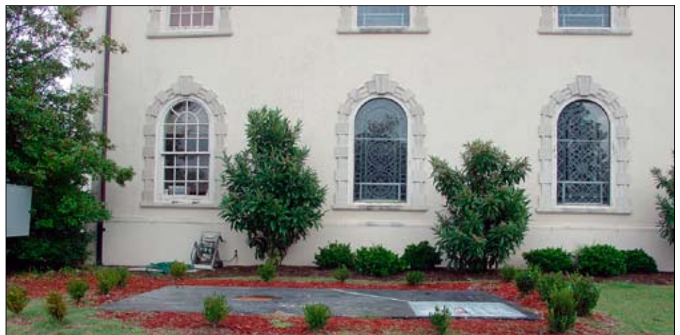
Fort Bragg's Main Post Chapel after the installation of a below-grade vaulted storage tank. This installation prevented a potentially costly heating fuel release and preserving the Historic District's integrity. With this discreet placement, all that can be seen from the street is a manhole cover and the strategically placed landscaping that surrounds the vault area.
