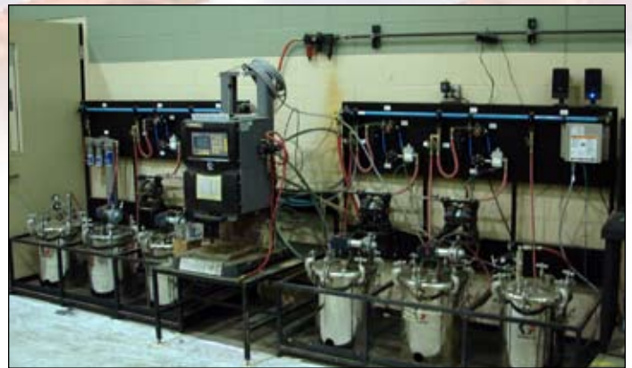
New paint mixers ensure the most efficient mixing and storage for vehicle and equipment paint. This not only reduces the likelihood of spills, but also simplifies operations for CSMS painters. Paint mixers also reduce waste by keeping paint fresh, avoiding the disposal of unused paint.
