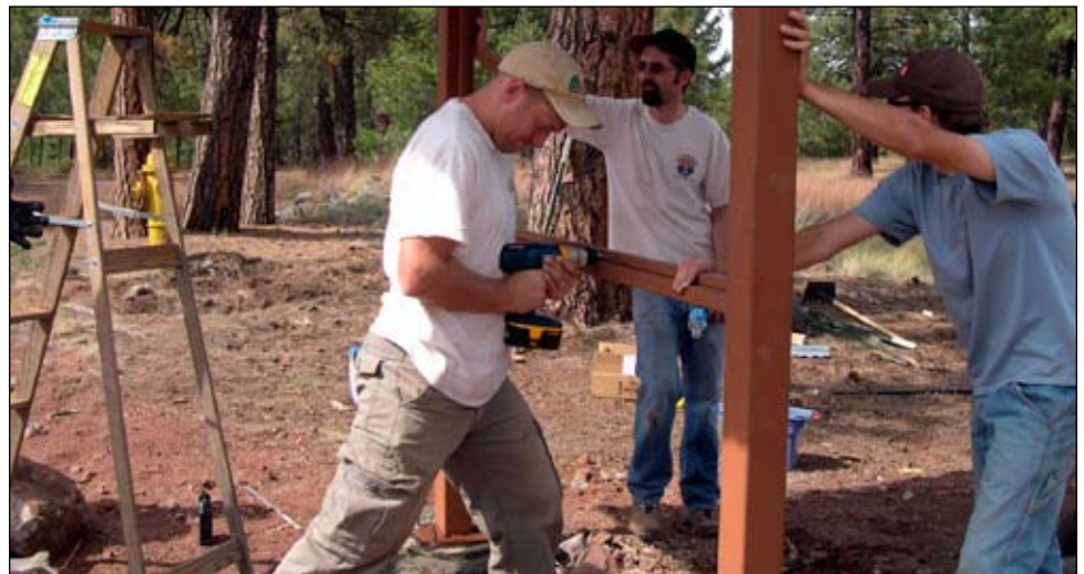
This 2007 photo depicts Dave Larsen, Tom Parker and Kevin Johnson constructing an interpretive kiosk at Camp Navajo. The kiosk was made of welded steel posts set in place and secured with poured concrete footings. The corrugated steel roof was designed to protect the interpretive display from the ravages of severe weather. (Photo by Dorenda Coleman, AZ ARNG Environmental Staff)
