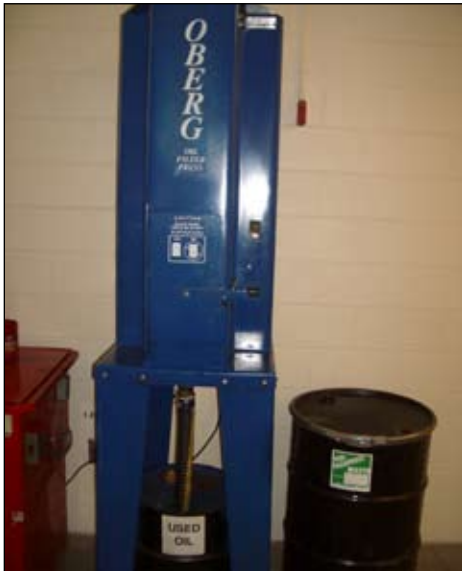
Fuel and oil filter crushers are part of recycling efforts at FMS 2. The crushers allow the P2 Team to reclaim petroleum products for recycling and allow used filters to be recycled as scrap metal rather than disposed of as hazardous waste. Antifreeze is also recycled with help from an outside recycling vendor.
