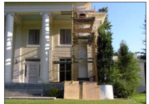
The Fort Drum CRM team plays an active role in responsible management of the LeRay Mansion Historic District. The team provided all of the preservation coordination for replacement of a deteriorated column at the Mansion and insured that the project met the Secretary of Interior standards. The team documented the unique column architecture and curated samples of the very unusual curved bricks that were produced at Fort Drum Historic Site 1290, the Brick Clamp at LeRaysville. (Photo provided by Gary Head, DPW Fort)
