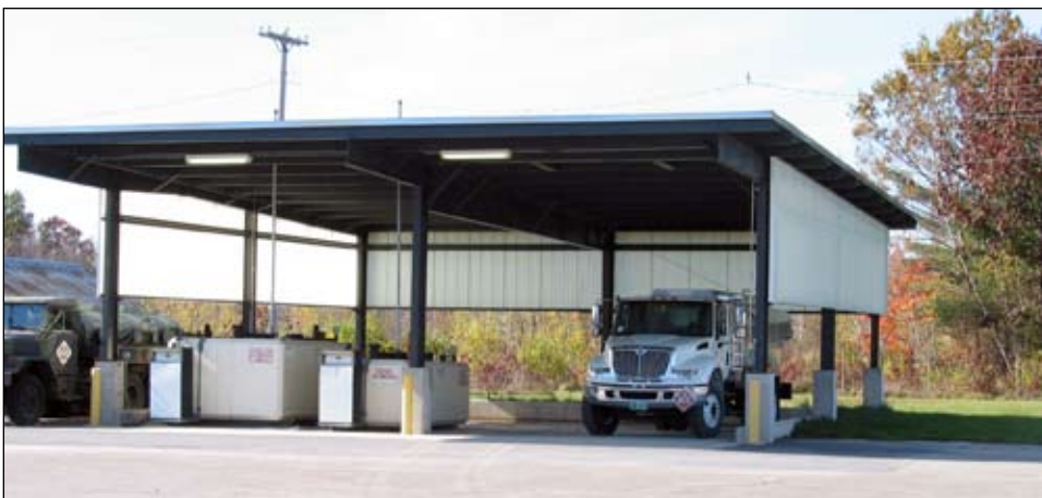
The Camp Johnson Fuel Point is a fully automated refueling station. Each vehicle has a key that operated the pumps and the pumps send the gallons used, mileage, and employee that pumped the fuel to a central computer. This fuel point is also a secondary containment not only for the tanks but for fuel transport vehicles when they are loaded.
