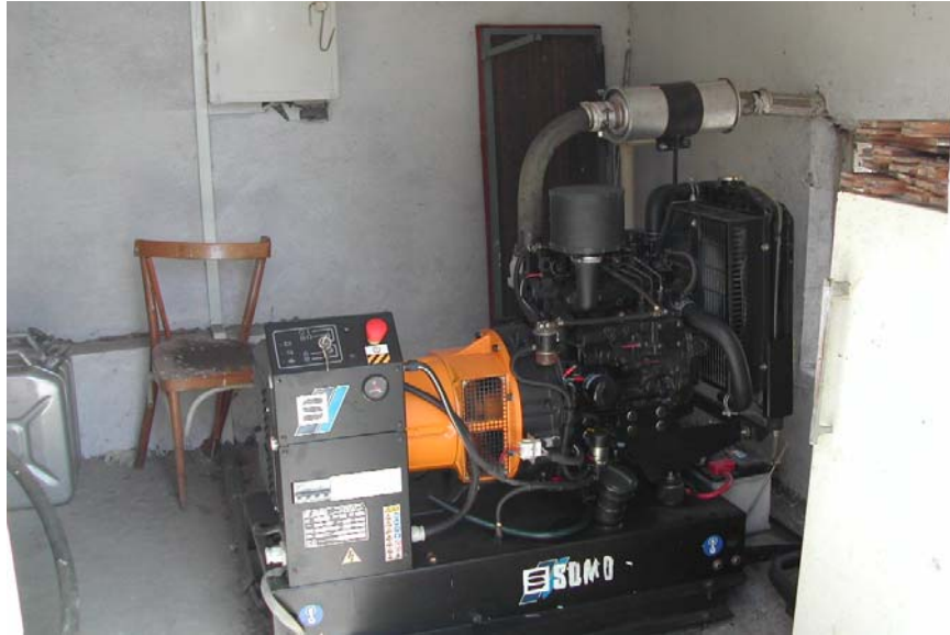
Photograph 3 This AIHA and USAID sponsored generator was an essential piece of equipment for the Mtshketa primary health care center since the city is frequently without electric power.
