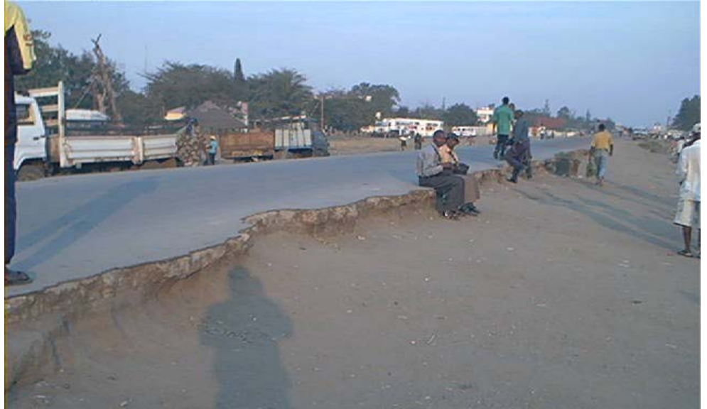
Photograph of a section of the EN205 road segment between the towns of Chokwe and Macarretane in Mozambique that was damaged by the floods. This photograph was taken before the reconstruction work began. (Photo by Mission Personnel, August 2001)
