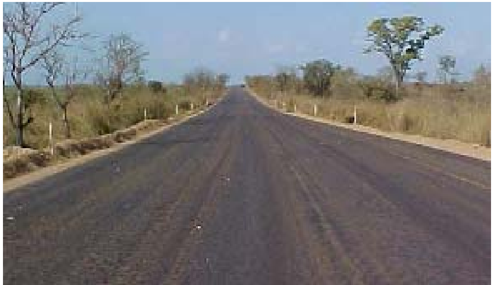
Photograph of completed section of the EN1 road segment between the towns of Gorongosa and Inchope in Mozambique. (Photo by RIG/Pretoria, August 2002)
