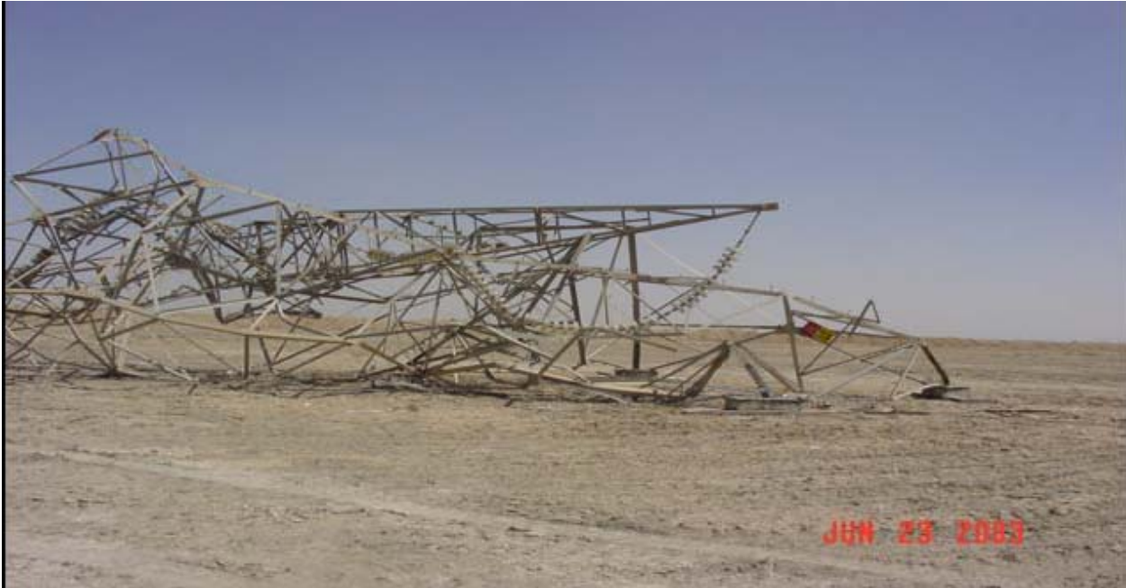
Photograph showing one of the 155 severely damaged transmission line towers along the Khor Al Zubayer-Nassiriyah corridor. USAID funded a project to refurbish these towers to permit the transmission of electricity through this corridor. (Photo furnished by Bechtel; undisclosed location in Southern Iraq; June 2003)
