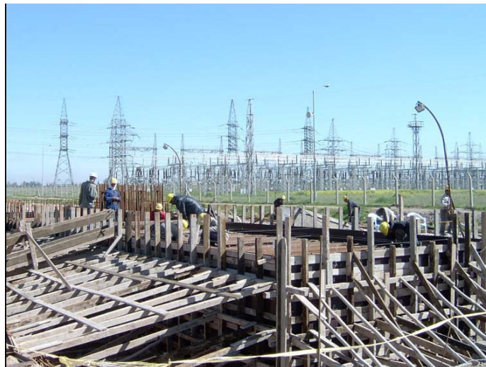
Photograph of the construction of the platform for one of the electric generation plants. (March 9, 2004)
