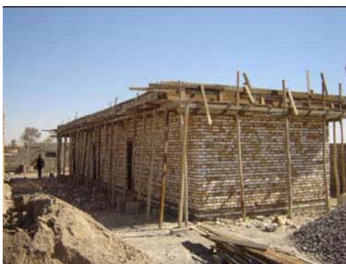
CAP II-funded construction of a school in an area experiencing an influx of displaced families. Source: USAID/Iraq.
