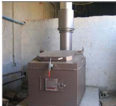
Prior to the provision of this CAP II-funded medical waste incinerator, hazardous hospital waste was mixed with general community waste. Source: USAID/Iraq
