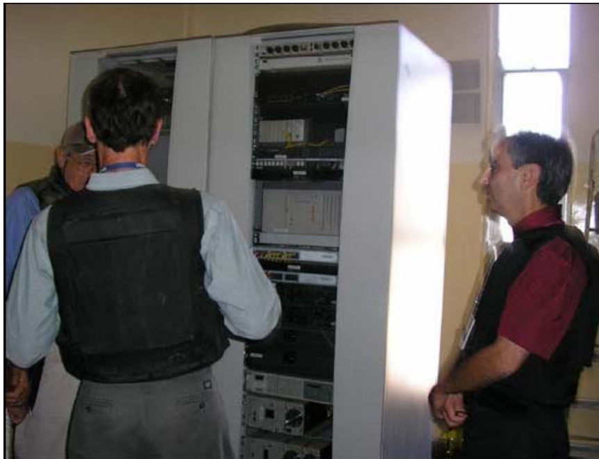
Photo of consolidated fiber network equipment at a power plant. The tower on the left is the operator. The tower on the right is the data receiver. (Central Iraq - September 2006)
