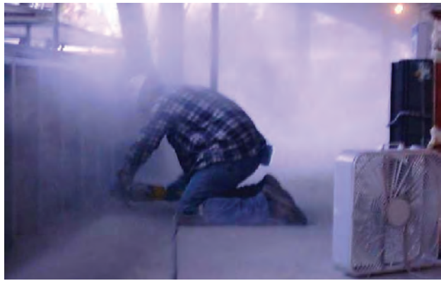
Using a grinder in poorly controlled conditions. (Photo courtesy of OSHA Directorate of Construction.)
