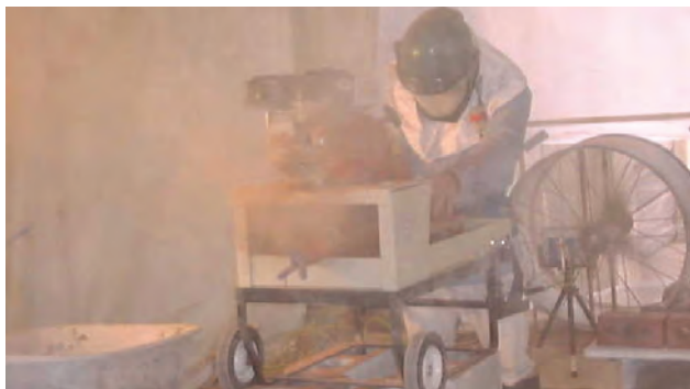
Hazardous exposures to silica can occur when stationary saws are operated without appropriate dust controls. (Photo courtesy of the University of Washington.)
