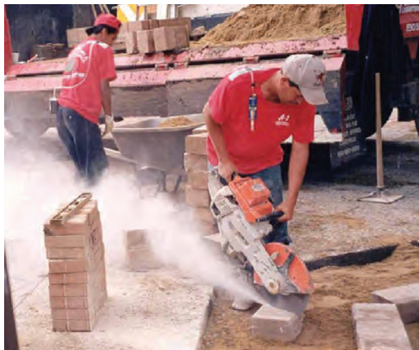
Employee operating a handheld masonry saw without the use of appropriate dust controls. (Photo courtesy of OSHA.)
