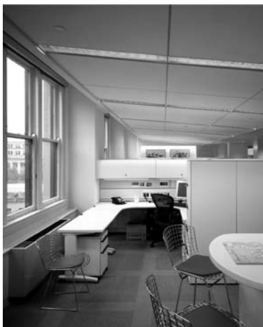
FIGURE 11 Preserve window opening clearance by recessing suspended ceilings from windows or configuring ceilings to slope upward toward the window head or step down toward the building interior.
