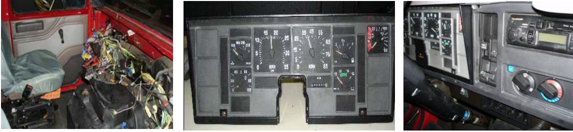
Figure 3.10: Cabin instruments wiring, dashboard gauges and instrument panel
