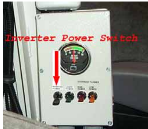
Figure 12. Photo. Remote switch for inverter power.
