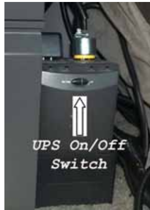
Figure 10. Photo. UPS on/off switch.
