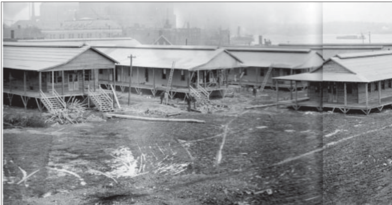
Figure 4.19. Panoramic photograph. This image is paired with Figure 4.20 to the right, depicting conditions during construction of General Hospital #2. General Hospital #2, Fort McHenry, Balto., MD. J. Henry Miller, Inc. Contractor, #57, 15 March 1918. Fort McHenry Library Special Collections, FOMC #2348.
