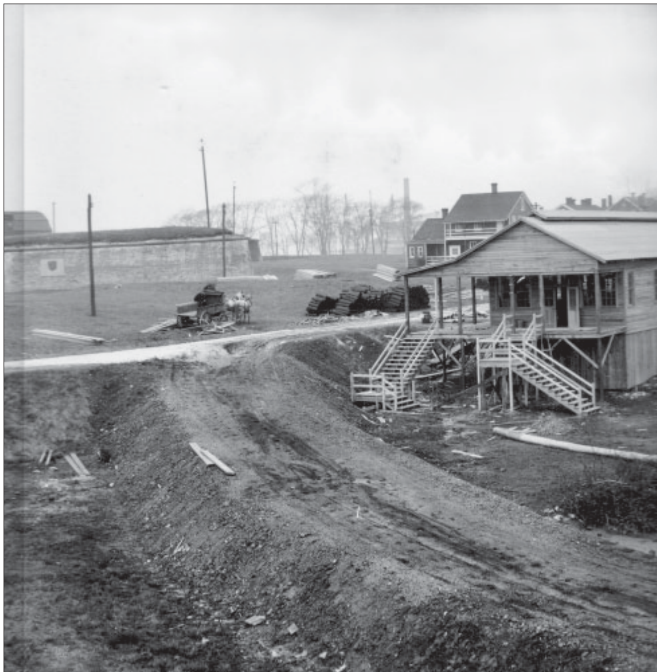
Figure 4.22. Panoramic photograph. This image is paired with Figure 4.21 to the left, depicting landscape conditions during construction of General Hospital #2. General Hospital #2, Fort McHenry, Balto., MD. J. Henry Miller, Inc. Contractor, 1918. Fort McHenry Library Special Collections, FOMC #2347.
