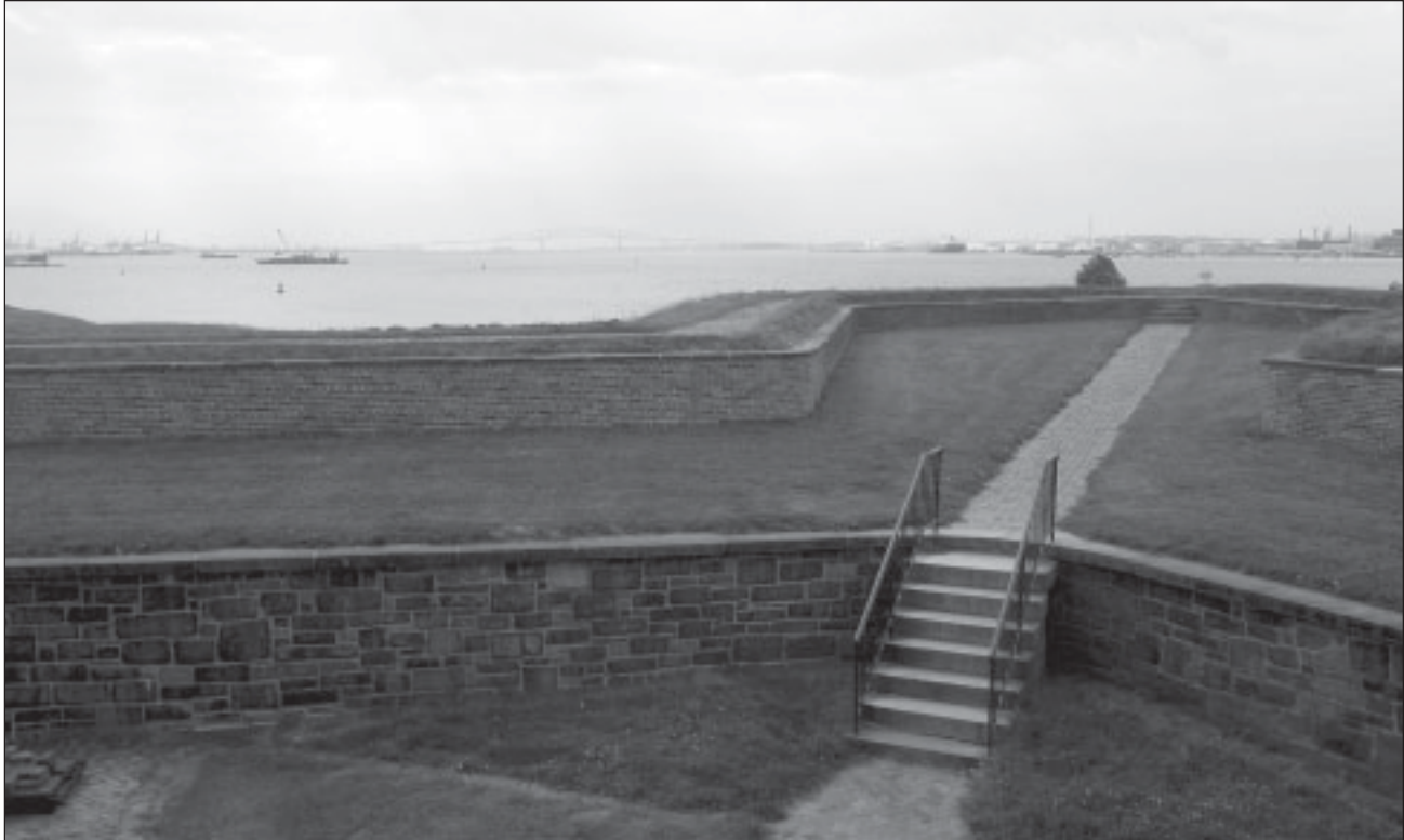
Figure 8.17 Star Fort Ramparts. Construction of the Star Fort Ramparts began in 1794; despite numerous repairs and alterations the configuration of the structure has been retained. The ramparts are comprised of several structural components constructed variously of earth and masonry. In profile these exhibit an irregular stepped appearance. Contributing. OCLP, July 2003.
