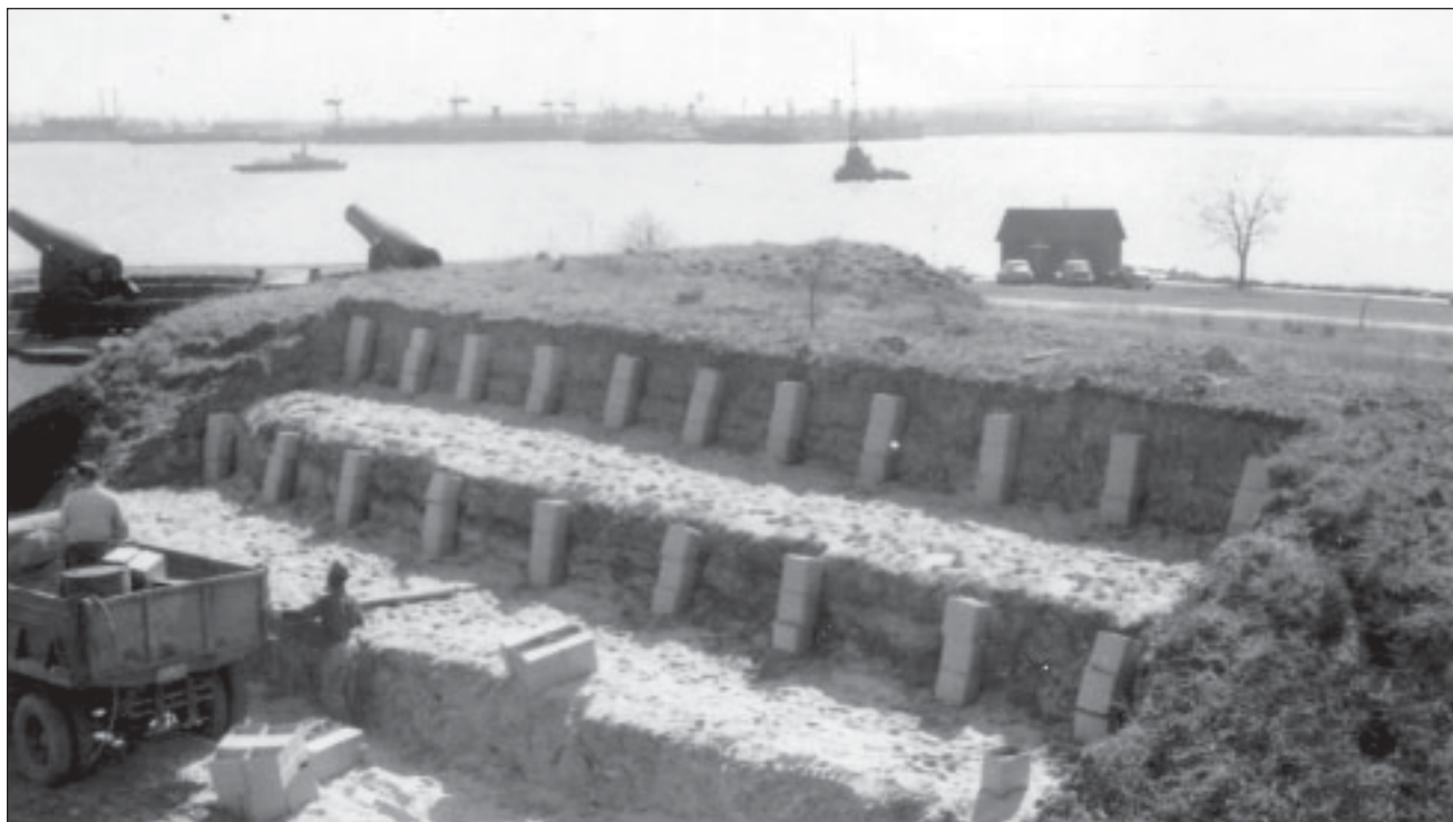
Figure 5.13. View of repairs and drainage improvements to fill covering Magazine 3, April 1950. This image shows the installation of interior drainage structures intended to reduce soil moisture. Small building at upper right is thought to be a temporary construction office. From, "Final Report on Repairing Slides in the Outer Ramparts..." 9 May 1950. Fort McHenry Library Special Collections.
