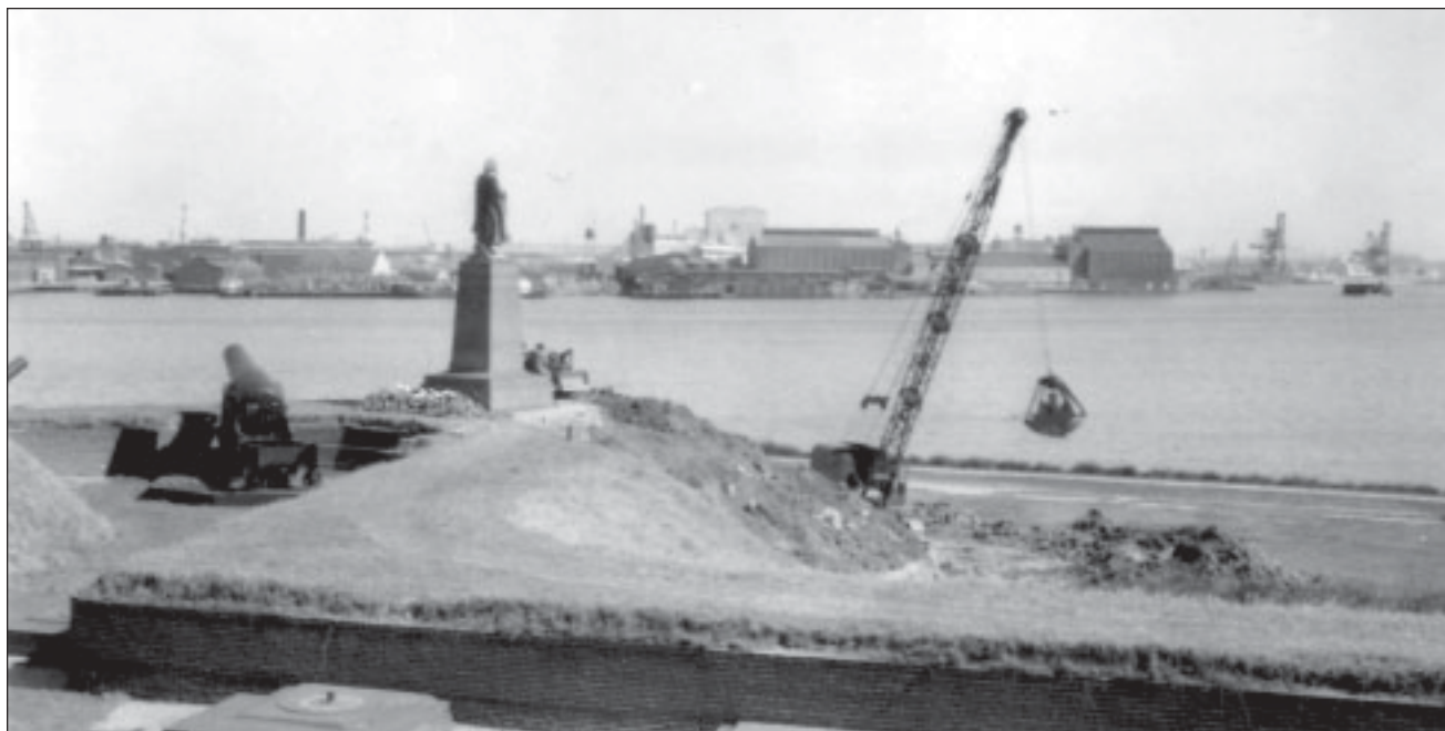
Figure 5.12. View of repairs underway to slope of exterior battery, April 1950. From, "Final Report on Repairing Slides in the Outer Ramparts..." 9 May 1950. Fort McHenry Library Special Collections.
