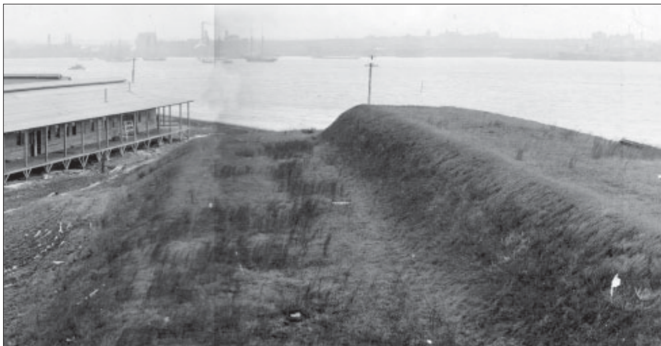
Figure 4.20. Panoramic photograph. This image is paired with Figure 4.19 to the left, depicting conditions during construction of General Hospital #2. Note unfinished water battery begun during the 1870s. General Hospital #2, Fort McHenry, Balto., MD. J. Henry Miller, Inc. Contractor, #57 15 March 1918. Fort McHenry Library Special Collections FOMC #2348.
