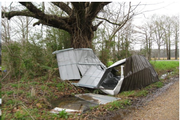
A shed was destroyed and blown across a road by an EF0 tornado in the community of Bodoc, Louisiana on February 21, 2008 (photo by Sam Shamburger, forecaster)
