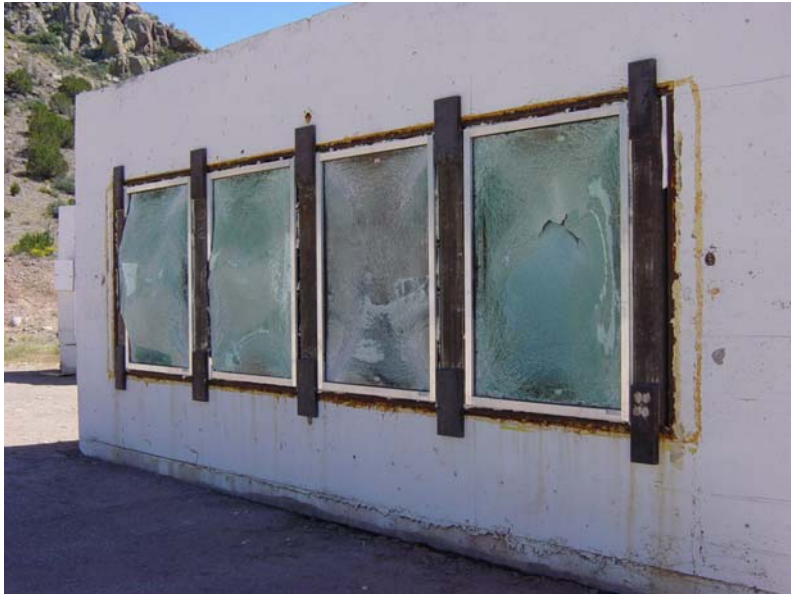
Figure 8. Post-Test Photo of Thick Laminate Window System Response.
