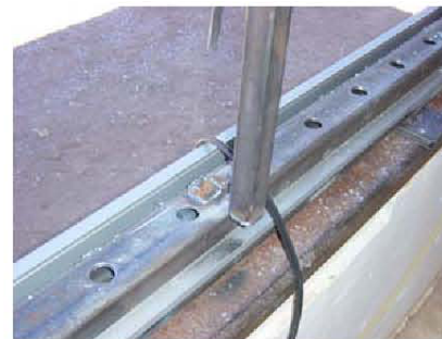
Figure 6. Failure of Standard Muntin End Connection.
